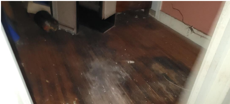
Figure 12. Interior – Water Damaged Wood Floor in 2023
