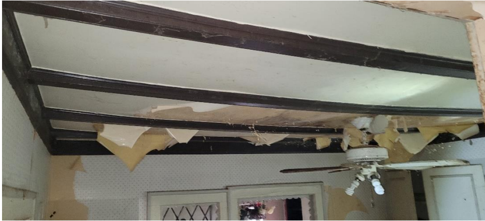
Figure 16. Interior – Water Damaged Ceiling in 2023
