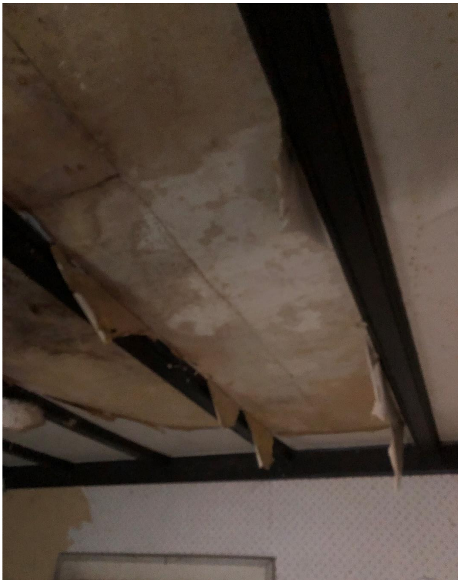
Figure 17. Interior – Water Damaged Ceiling in 2023
