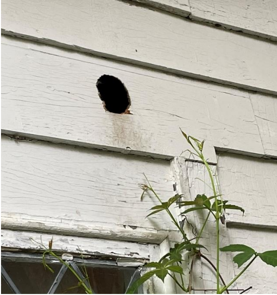
Figure 26. Hole in Clapboard on Side (East) Elevation in 2024
