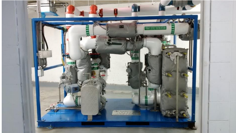
Figure 26: Space Heating and DHW ETS Skid 7
