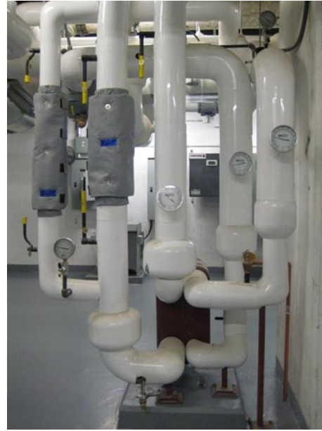
Figure 5: Typical ETS Installation 5
