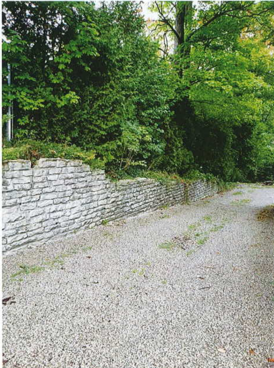
View looking down driveway at wall from Westwood street side with chain-link fence post (property line) visibly embedded in common boundary area
