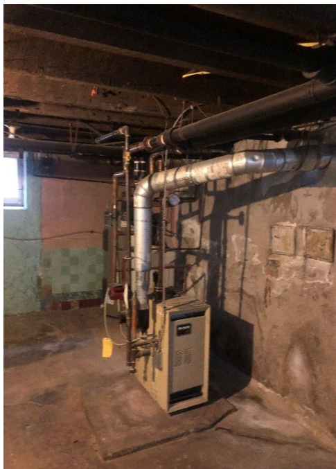
Fig. 05 Photograph of existing mechanical systems.
