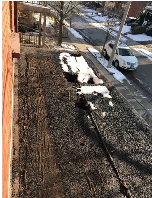
Fig. 02 Photograph of the existing balcony.
