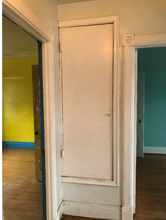
Interior – Remove the closet door to the existing stairs to the attic.
