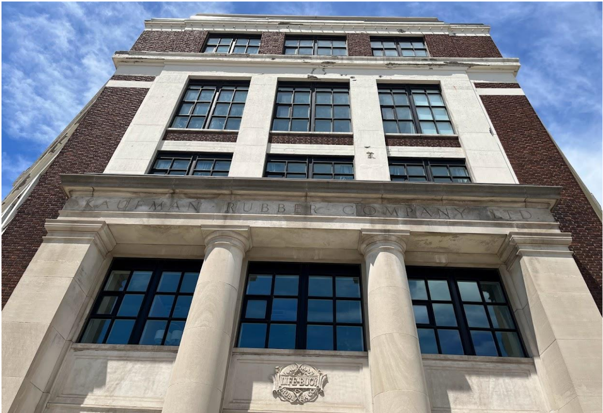
Figure 5: 404 King Street West Before Repair Work
