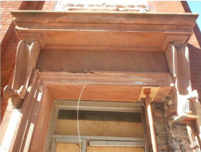
Detail photo showing cracked top portion of entrance surround and broken scroll.
