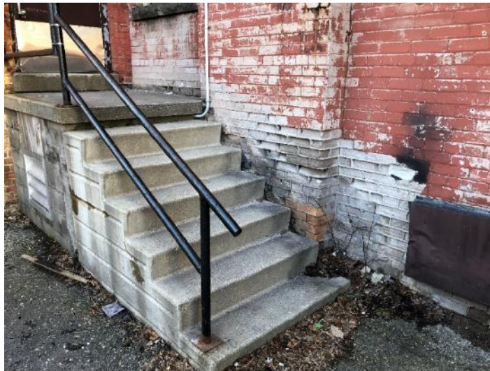
Deterioration of mortar joints and masonry units
