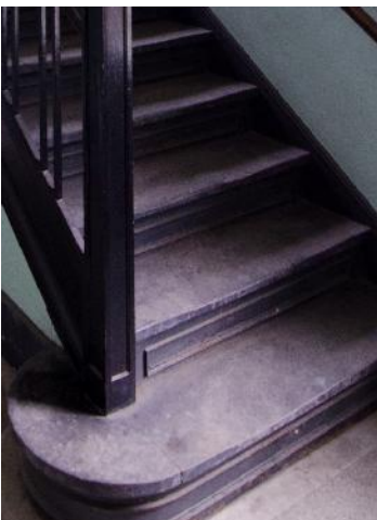
Detail photo of metal risers.
