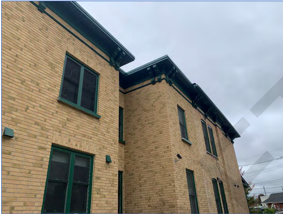
Photo 2: Detail showing transition between original building at 115 Water Street North (right) and two-storey addition (left) constructed in 2020
