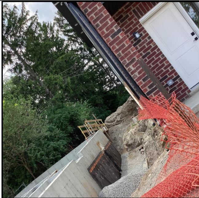
Figure 5: The west side yard where the 1.1 metre sidewalk will be still under construction
