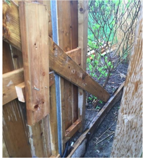
Above Right: A 1x6 deck board was used as stringer instead of conventional 2x4 or 2x6 boards. Because it was too short, a random piece of lumber was joined to it by a diagonal board that also served as a brace.
