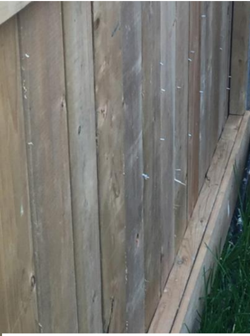
Above Left: Nails and screws protruded through the lumber.
