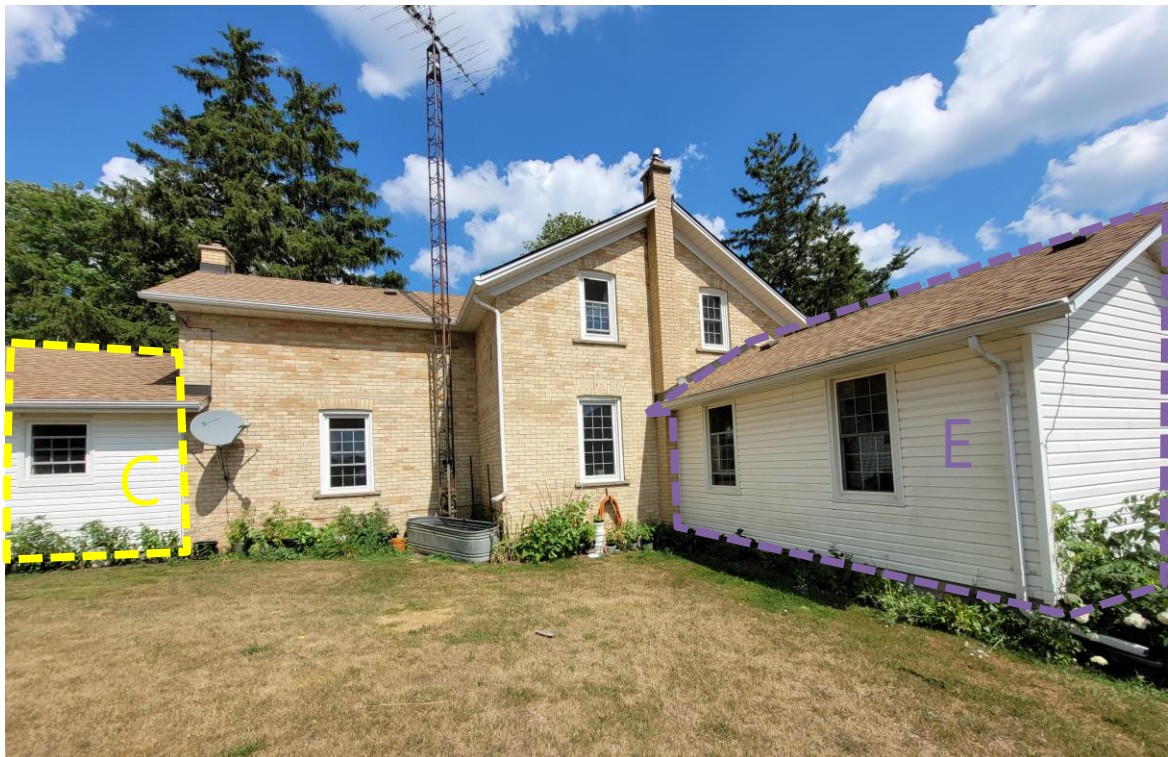
Figure 5: West Side Elevation with Contemporary Additions to be Removed Identified as "C" and "E"
