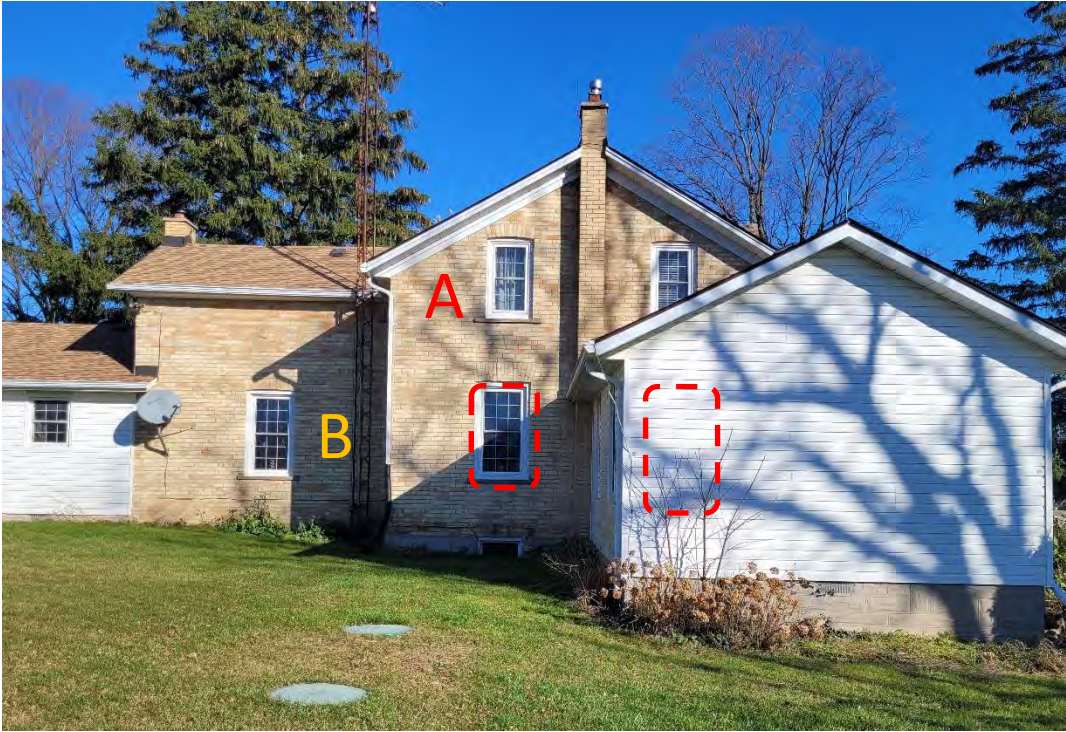
Figure 31: View of west elevation, looking north, noting location of door opening at the interior of the building (west wall of Section "A"). (Source: MHBC, 2023)
