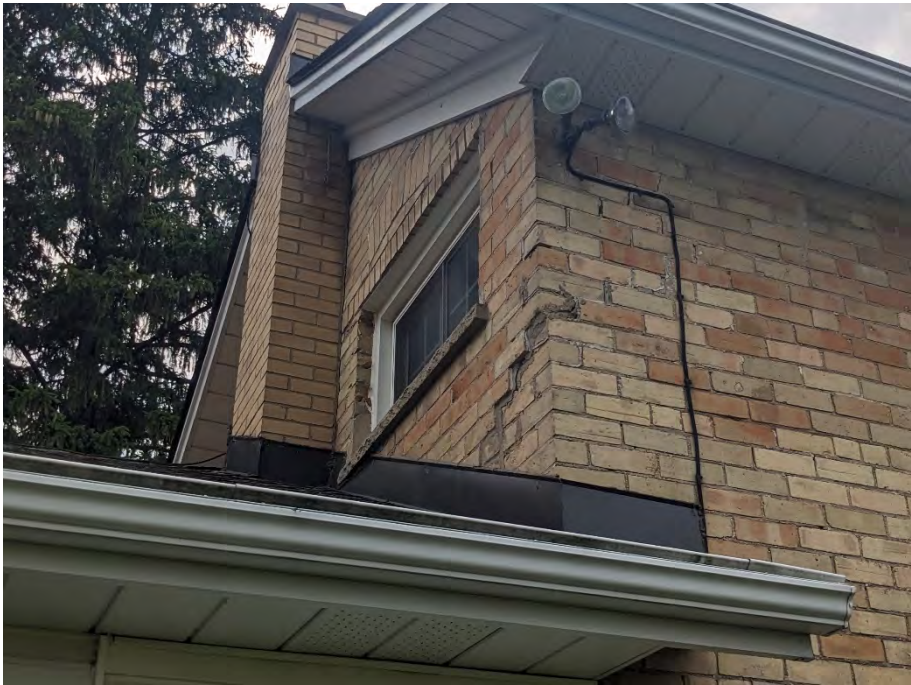
Photograph 2 – Damaged Corner Repaired with Cement
