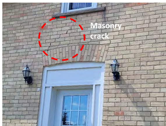
Figure 19: Example of step cracks over front elevation door.
