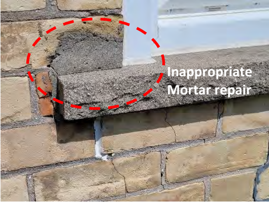
Figure 20: Example of inappropriate cement repair.
