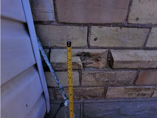
Figure 22: Example of broken bullnose brick.
