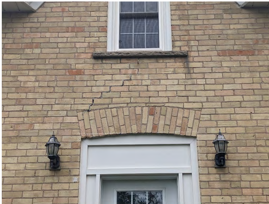
Photograph 1 – Step Cracks Over Door Opening
