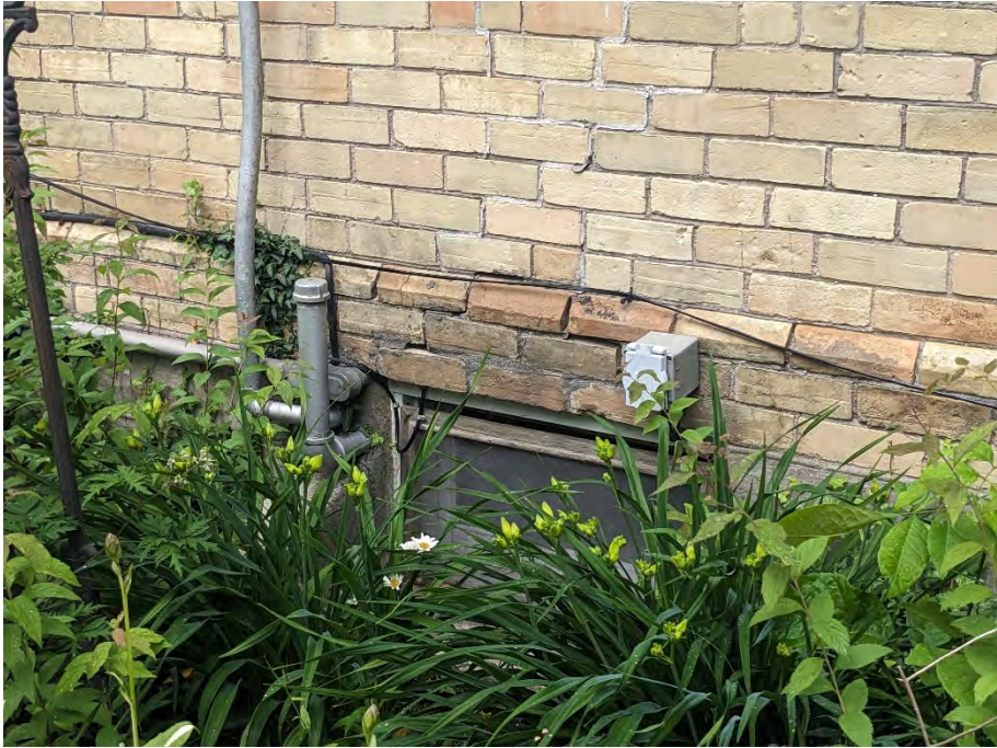
Photograph 3 – Joint Cracking and Sealant Repairs
