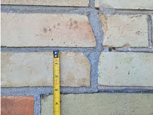
Figure 23: Example of inappropriate cement mortar repair.
