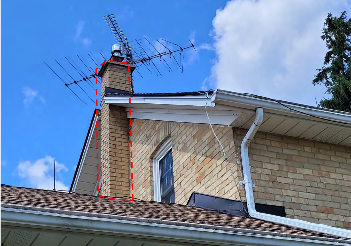
Figure 24: Detail view of existing chimney at south elevation, demonstrating different (contemporary) bricks and is not original to the structure (Source: MHBC, 2023)
