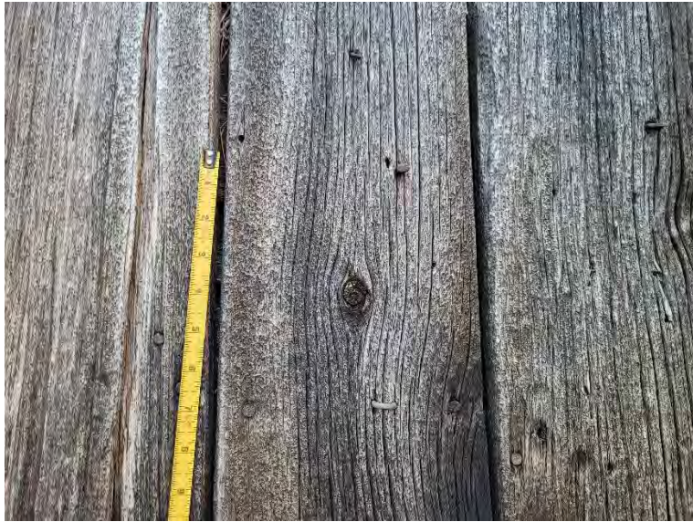
Figures 13 & 14: (left) Detail view of typical barn board cladding at east elevation, (Source: MHBC 2023)
