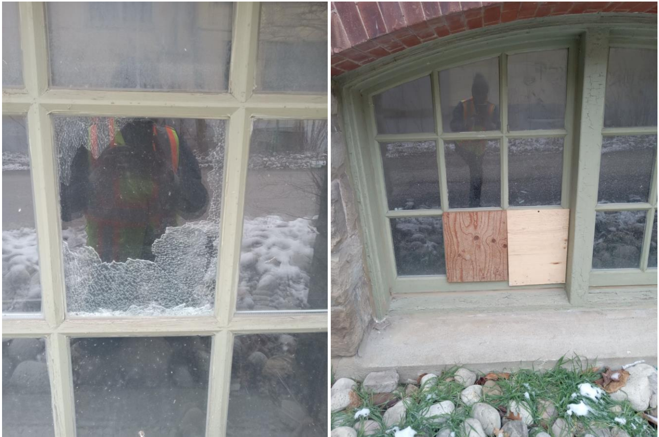
Figure 3-4: Broken Windowpanes on the Subject Property
