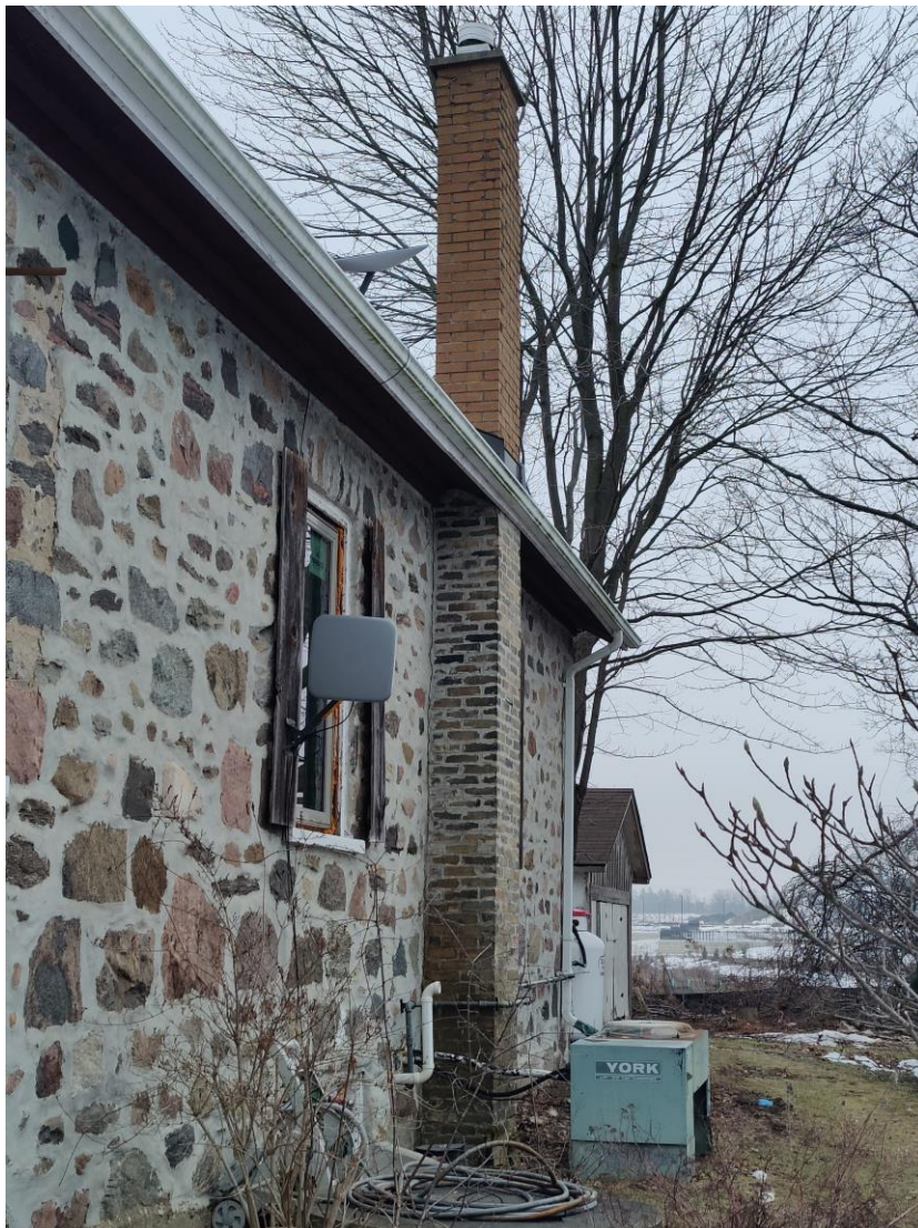
Figure 4. Current condition of the chimney on west façade.
