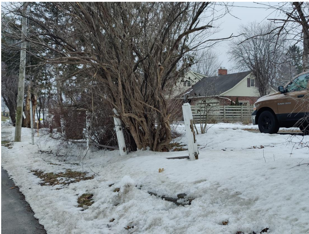
Figure 7. Rotting cedar and missing pieces on the fence.
