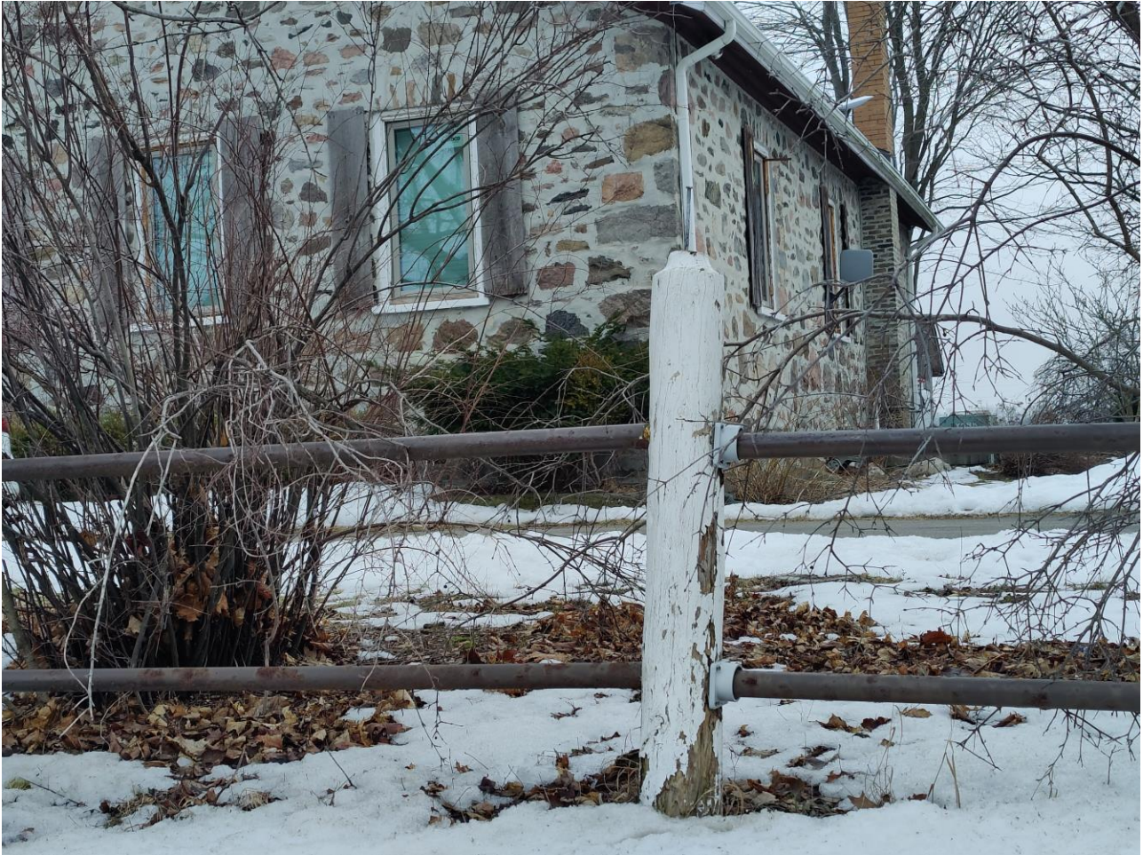
Figure 8. Missing tops on the fence.
