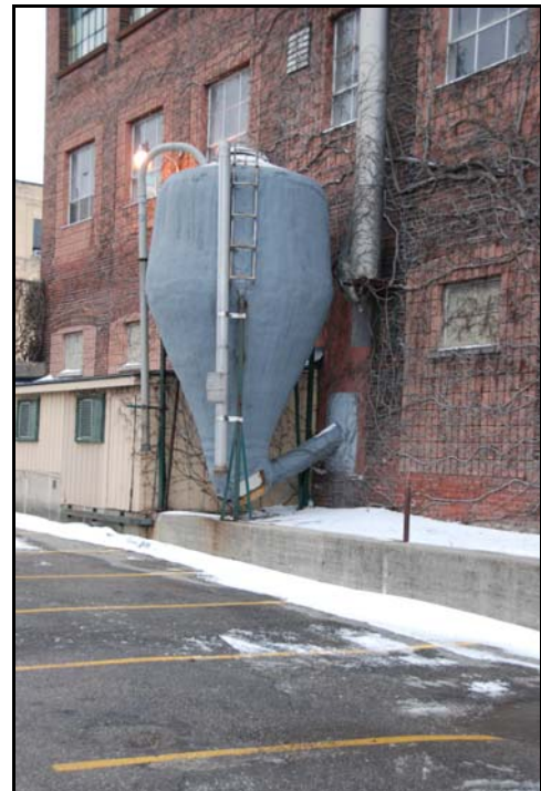
Figure 28 exterior salt system
