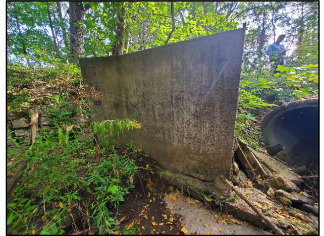
Photo 8. Damaged crossing downstream of Hidden Valley ESPA/PSW
