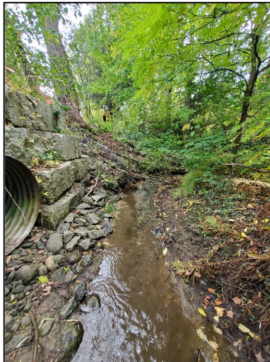
4. Hidden Valley road culvert. West side of Hidden Valley Road, looking south. Showing the location of the seep located immediately downstream of the culvert.
