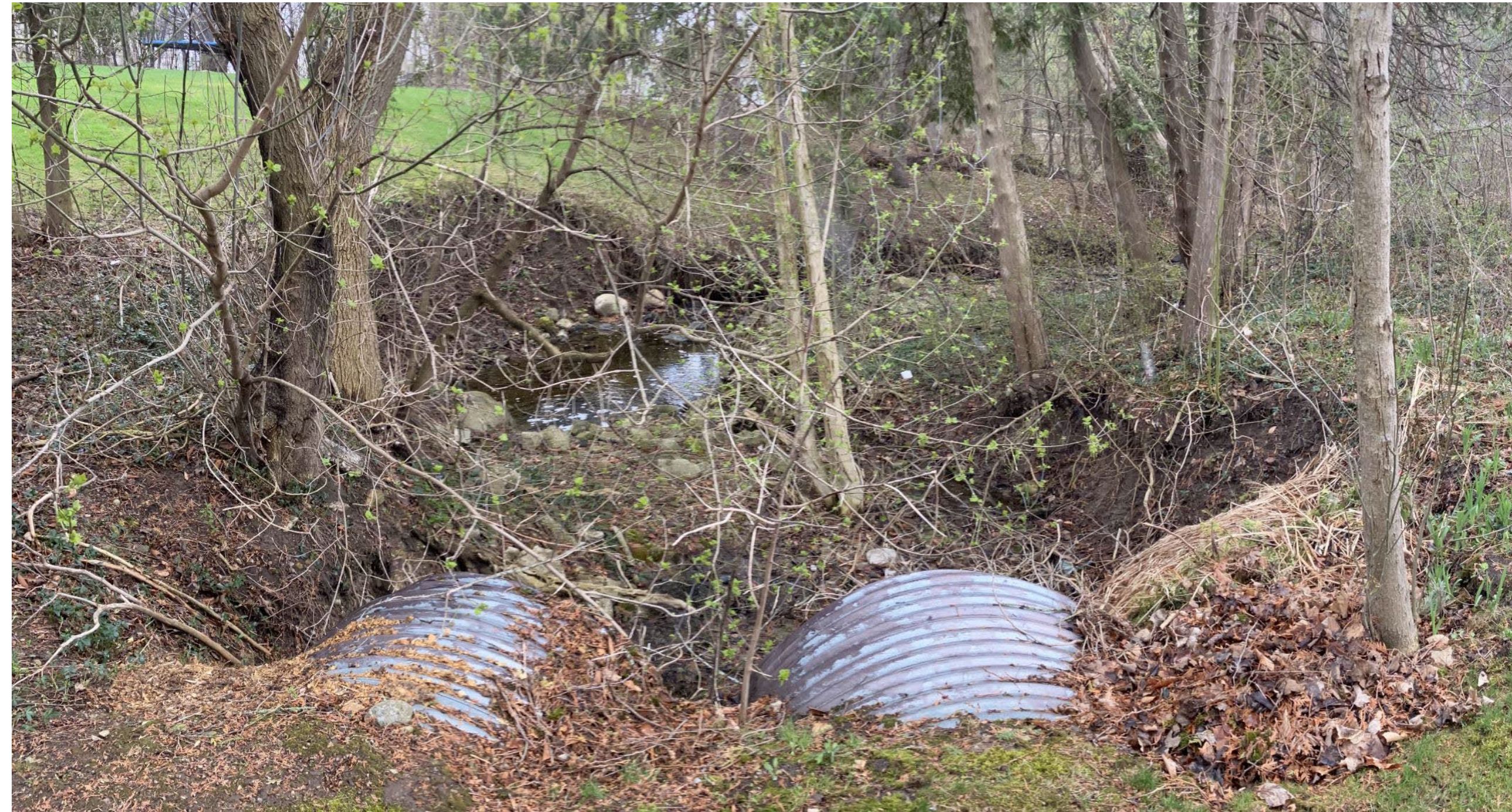
Erosion just upstream of Hidden Valley Road; potential source of material reducing capacity at road culverts
