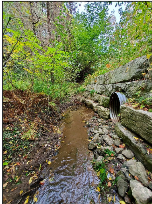
3. Hidden Valley road culvert. West side of Hidden Valley Road, looking north.
