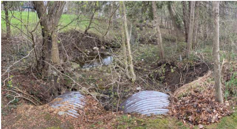
Erosion just upstream of Hidden Valley Road; potential source of material reducing capacity at road culverts
