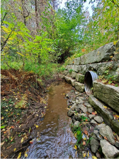
Photograph 1: Upstream view of Hidden Valley Road Culverts. The low flow culvert cannot be seen below the sediment.
