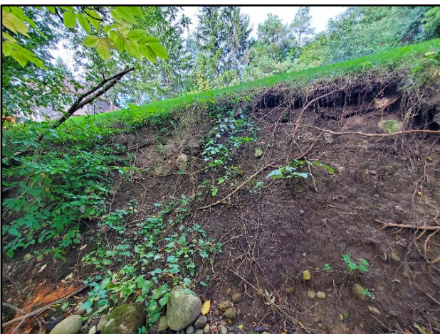
Photo 11. Erosion Noted upstream of Hidden Valley Road
