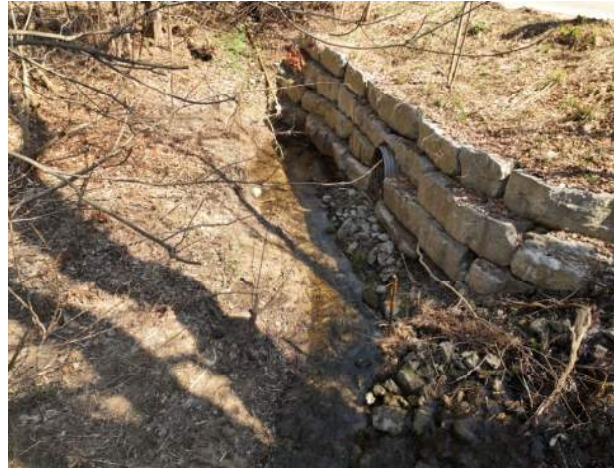
Headway of Hidden Valley Road crossing; note almost complete submersion of easterly culvert by sedimentation
