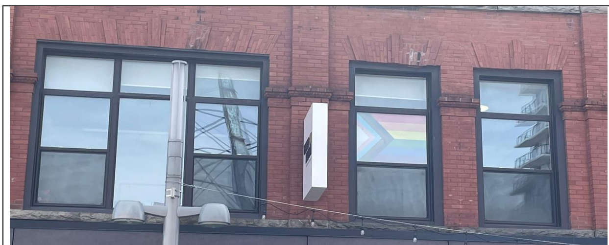
Detailing of second-storey with a ribbon of three windows in the first bay; two flat head window openings in the second bay; rectangular transoms; and, 1/1 hung window design with brick voussoirs and continuous stone sills
