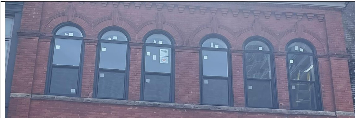
Detailing of second-storey showing semi-circular window openings; semi-circular transom; 1/1 hung windows; and, decorative brick hood moulds with keystones and continuous stone sills
