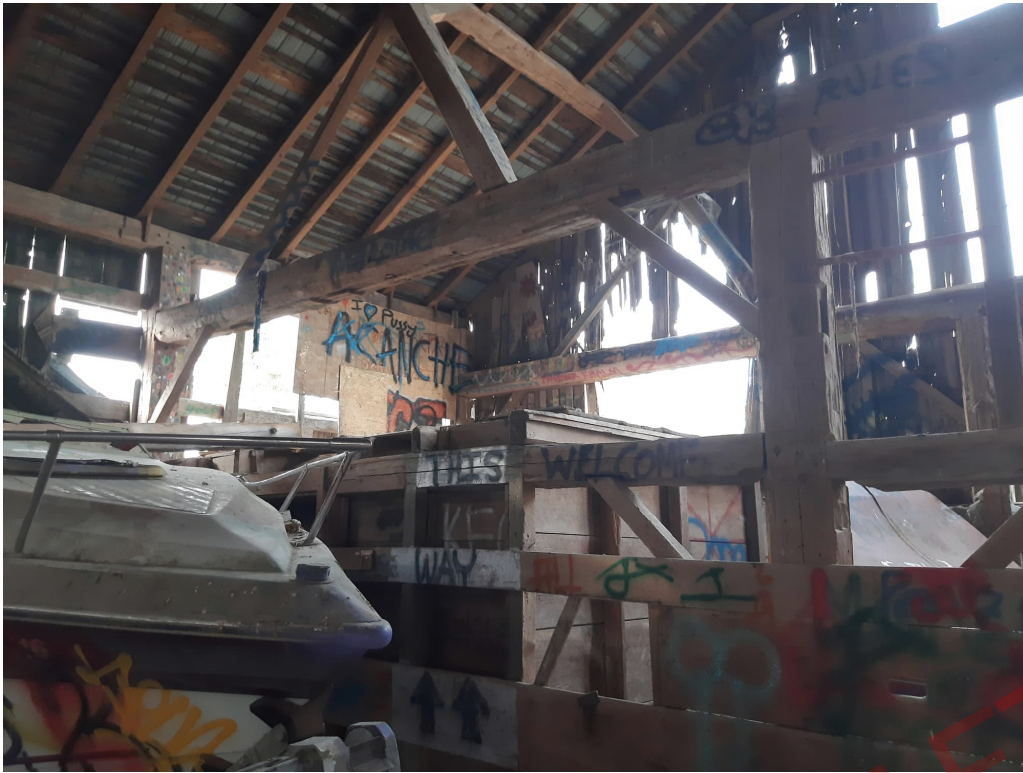
Photograph No. 1 – Missing Wall Cladding, Interior Framing Exposure to Elements
