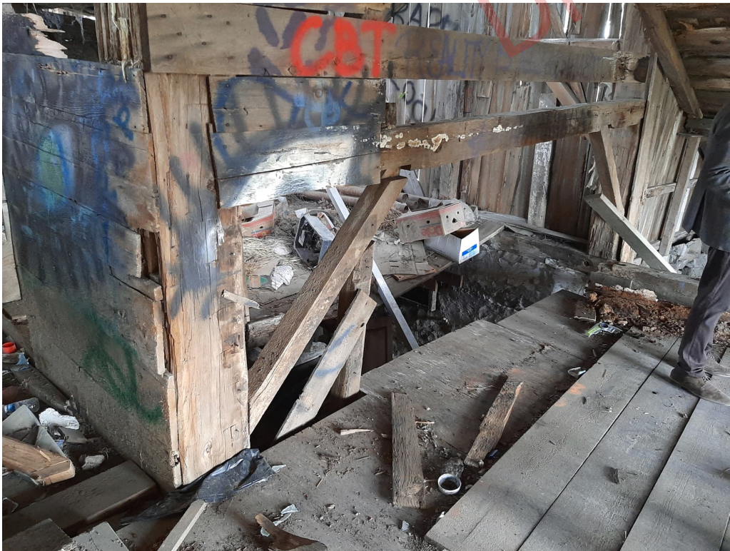
Photograph No. 2 – Compromised Brace Connection, Unsafe Open Floor
