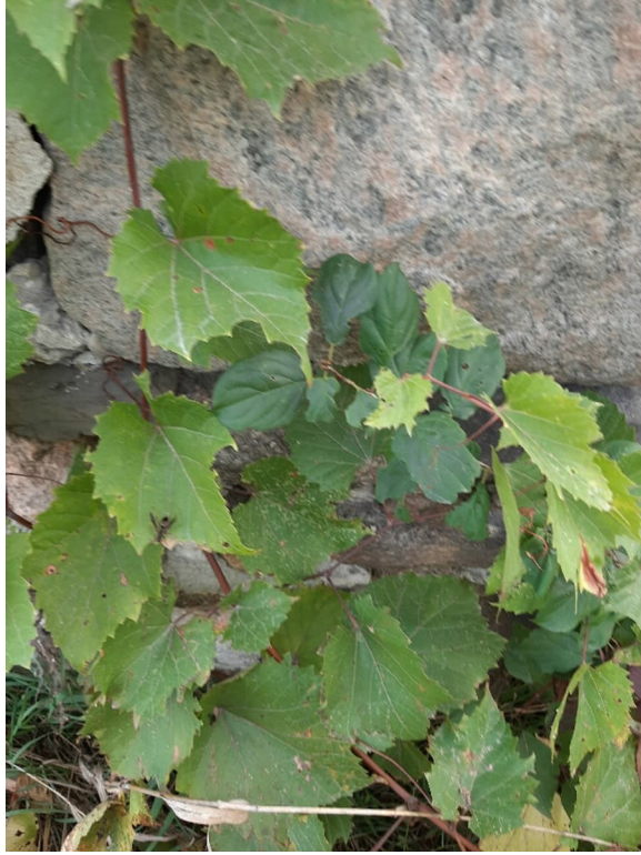
Photograph No. 13 – Stone Foundation Wall Deterioration
