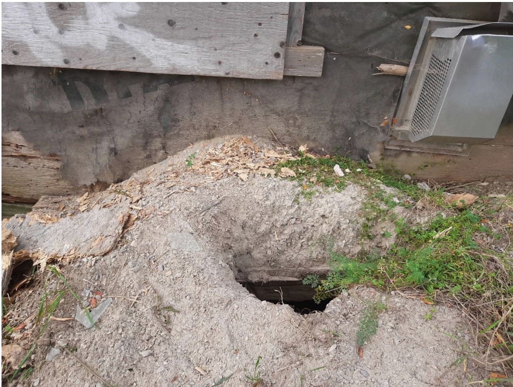
Photograph No. 15 – Soil Pile Causing Rot of Wood Framing
