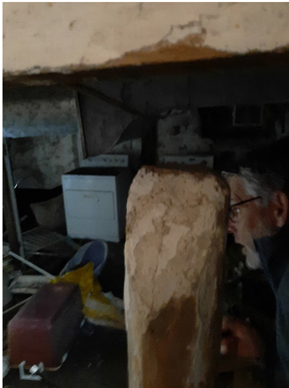
Photograph No. 21 – Loose Disconnected Support Post
