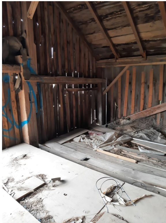
Photograph No. 8 – Unsafe and Unsecured Flooring
