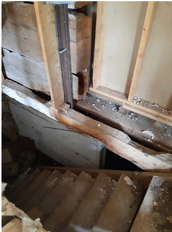
Photograph No. 17 – Stair to Basement - Rot of Bottom Wall Log
