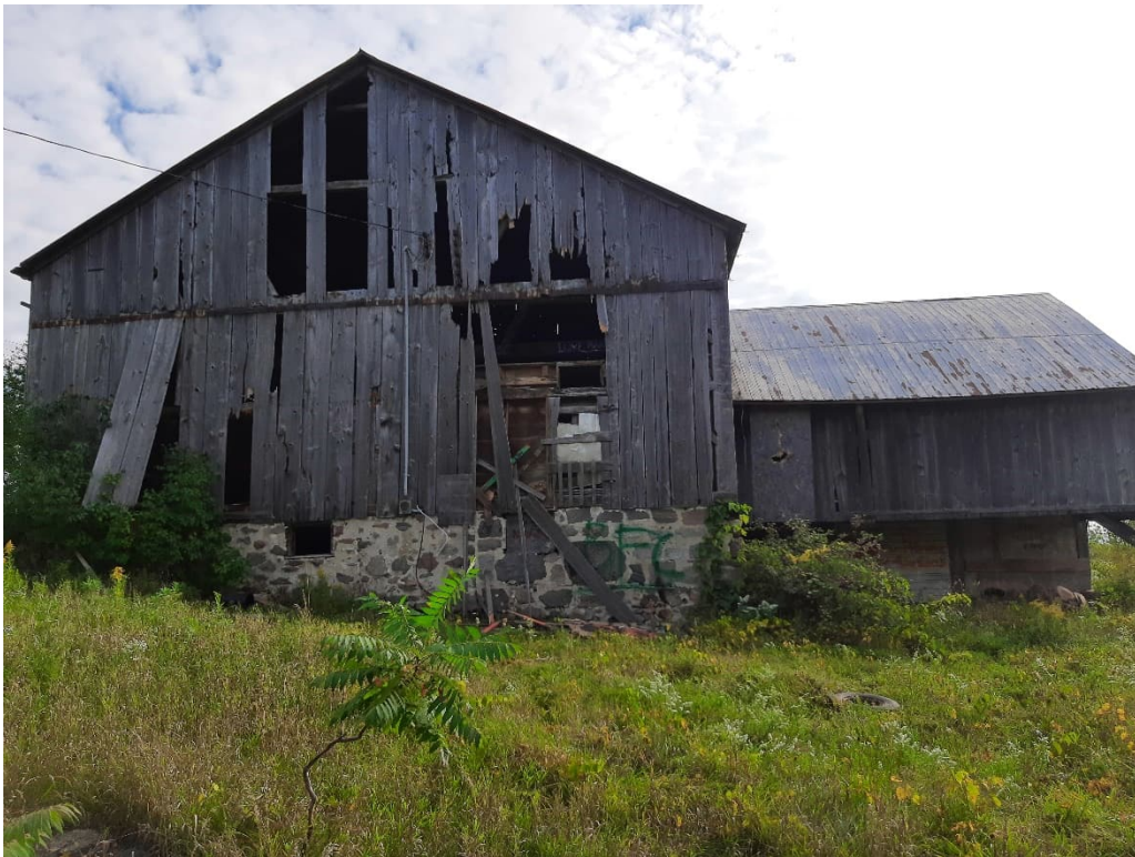
Photograph No. 12 – West Elevation; Wall Boards Missing
