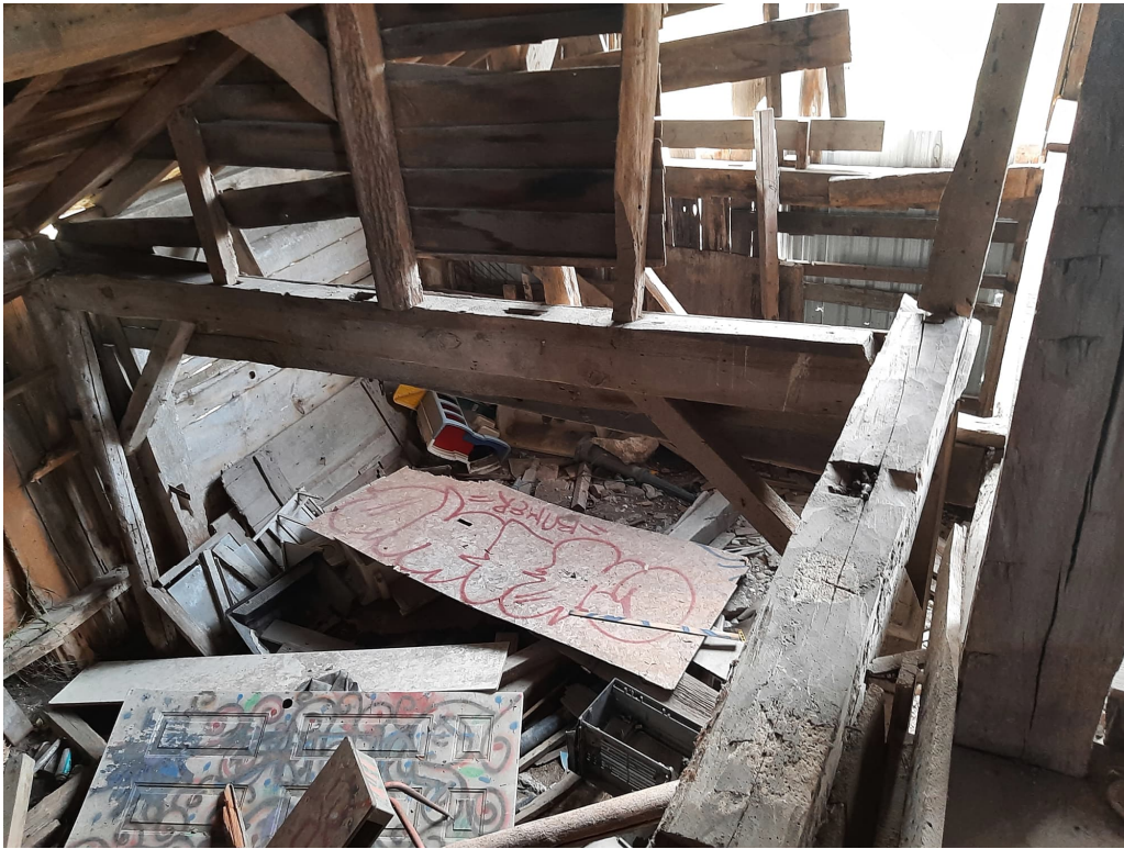
Photograph No. 7 – Deteriorated Framing and Connections
