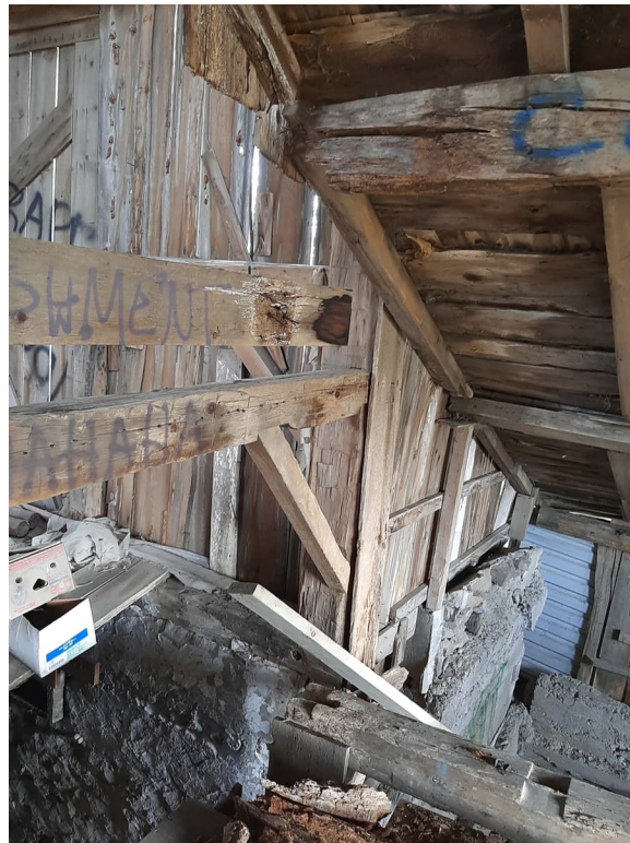
Photograph No. 4 – Post Missing, Unsupported Roof Beam
