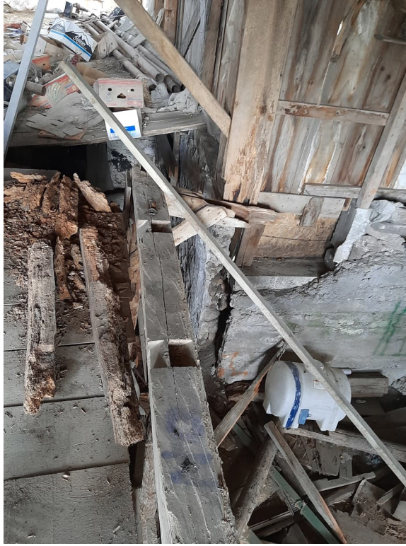
Photograph No. 5 – Unsafe Condition, Compromised and Deficient Bracing and Connection of Wall and Floor Framing
