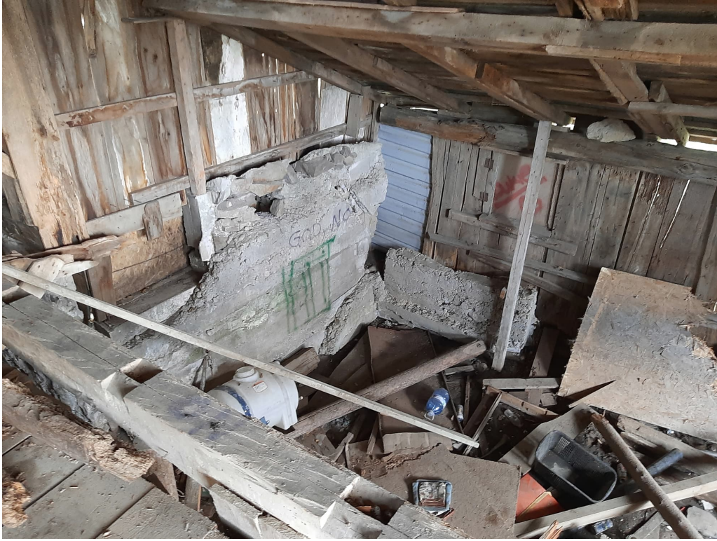
Photograph No. 3 – Unguarded Edge of Floor, Deteriorated Concrete Foundation Wall
