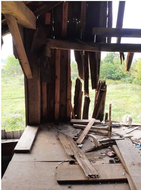
Photograph No. 6 – Unguarded Area, Missing and Deteriorated Wall Boards
