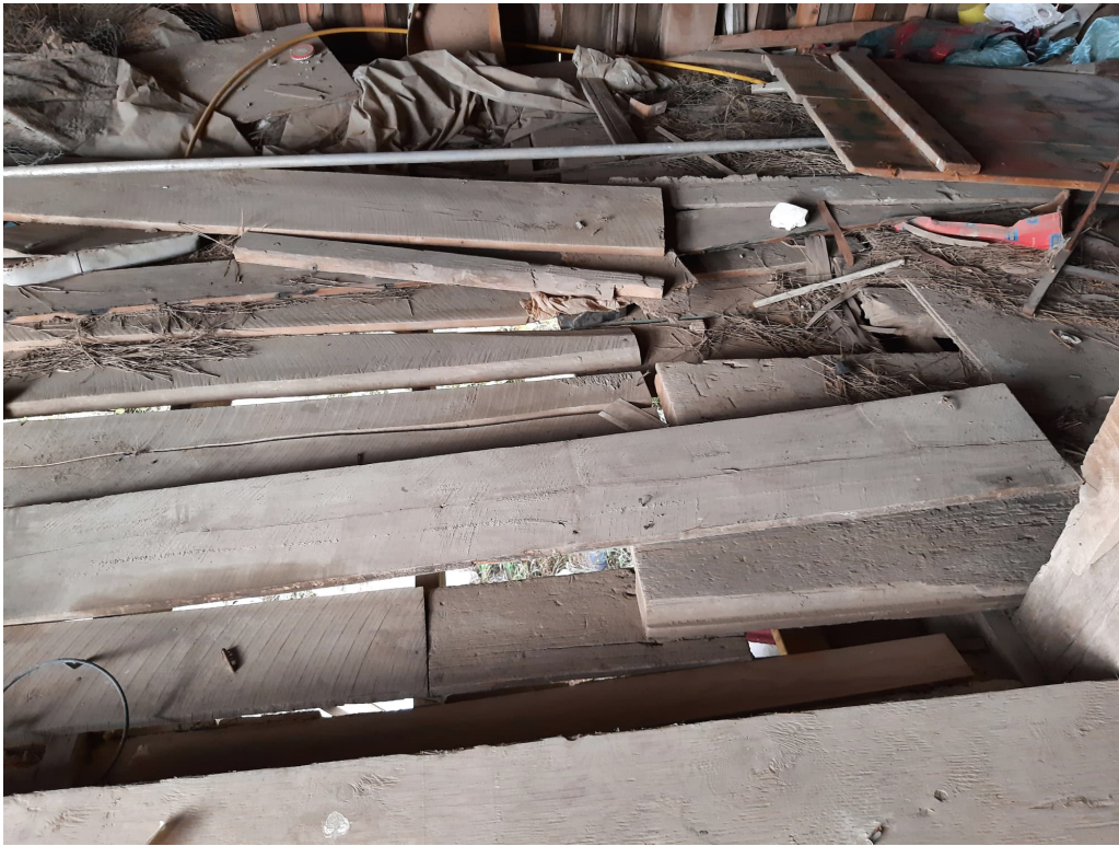
Photograph No. 9 – Unsafe Floor; Unsecured Flooring
