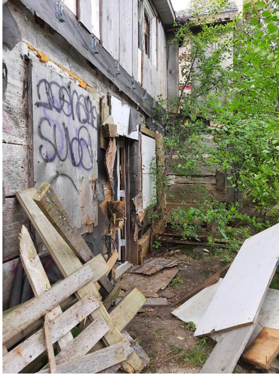
Photograph No. 16 – Unprotected Exposed Wall – Deterioration
