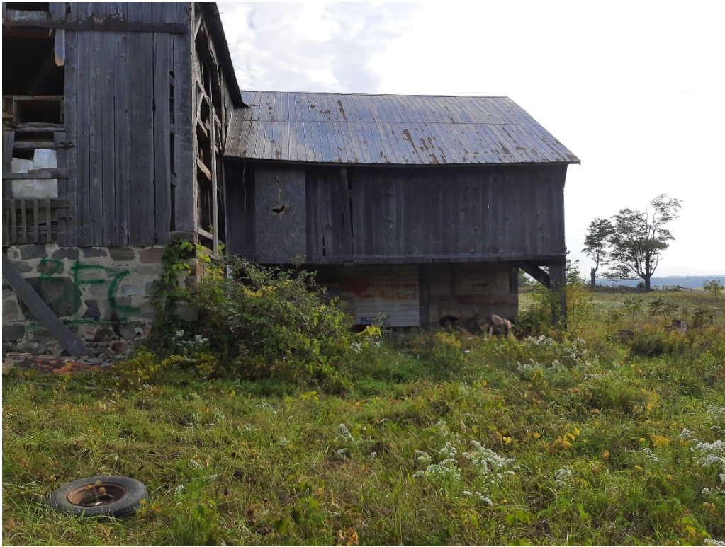
Photograph No. 11 – West Elevation; Building Sagging from Insufficient Support
