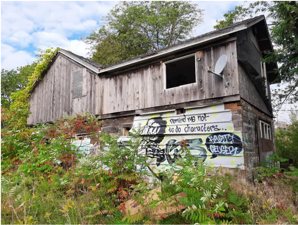
Photograph No. 14 – Overall Photo Of House
