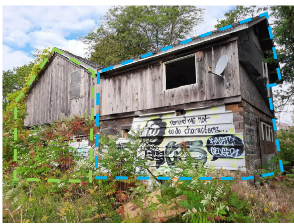
Figure 21: South elevation (rear façade), view is taken from the back of the house (MTE, 2023). Original dwelling noted in green, later additions noted in blue.
