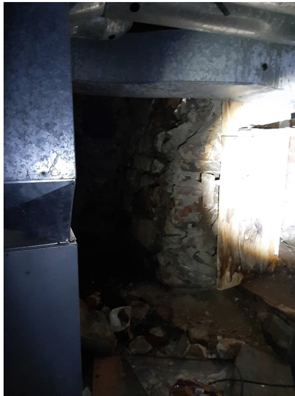
Photograph No. 19 – Basement Foundation Wall Mortar Deterioration
