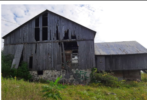
Figure 15: West elevation (side façade), view is taken from west side of property. West wall boards on missing on original barn portion (MTE, 2023)
