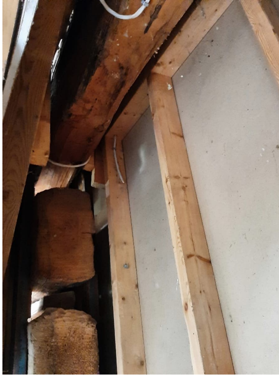
Photograph No. 22 – Upper Story Wall End Logs Unbraced (No Framing)
