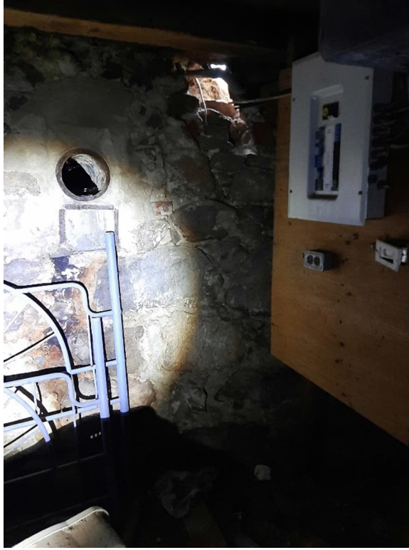
Photograph No. 20 – Foundation Wall Deterioration Open Window Well
