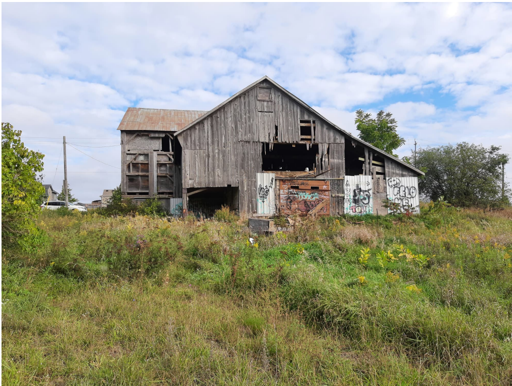
Photograph No. 10 – South Elevation Wall Boards Missing
