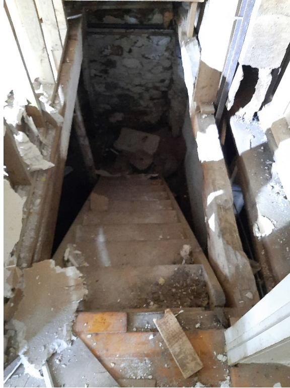
Photograph No. 18 – Stair to Basement; rot of log (right)
