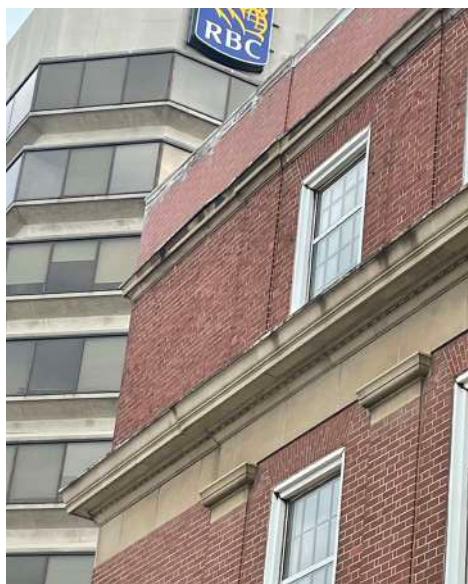
Figure 9. Detail of the front facade fronting Duke Street West. The parapet brick appears to have been replaced as variation in brick stain was observed. (Source: mCs, July 2021)
