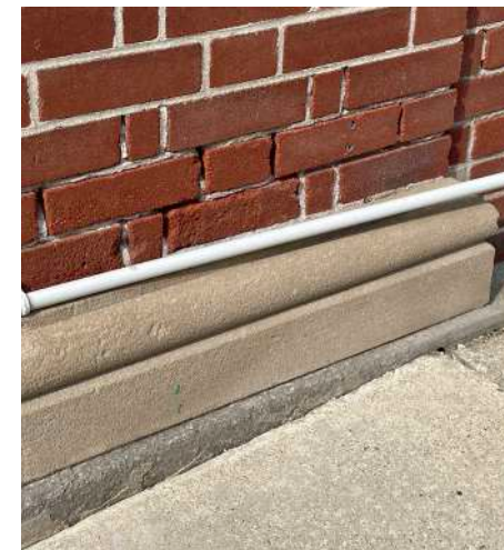
Figure 14. Poor repairs to masonry and mortar. Bricks should be repointed with mortar that is compatible with existing. (Source: mCs, July 2021)
