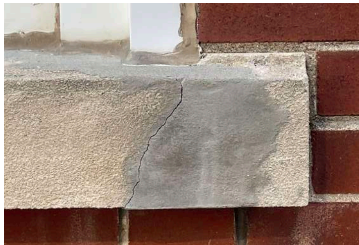
Figure 13. Cracking and deterioration in the sill. The repair is visually intrusive and measures should be taken to rehabilitate the sill to make it visually compatible to its original design. This inspection was undertaken with the naked eye and is not intended to identify any structural issues. (Source: mCs, July 2021)
