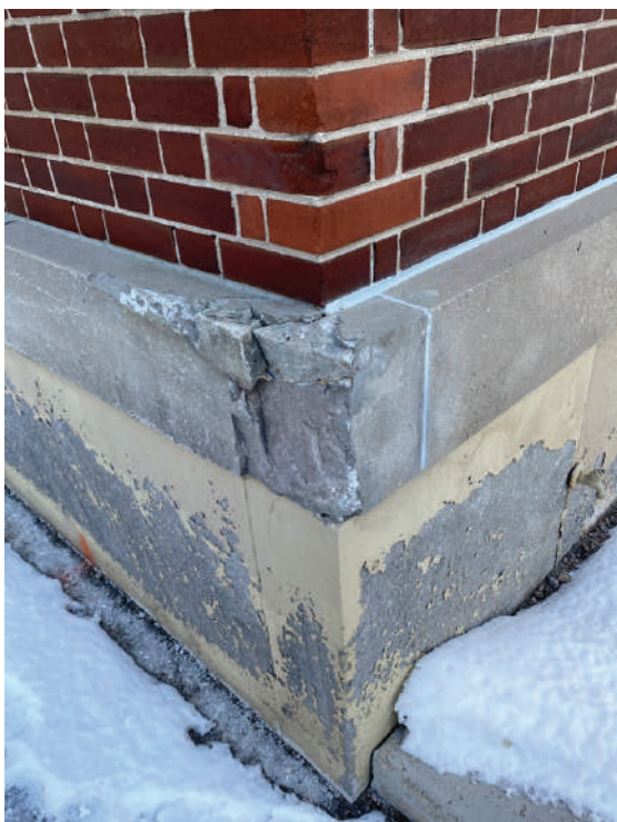
Figure 26. Damaged stone banding and bricks to repair.
