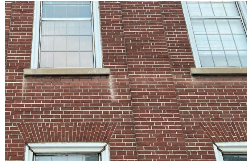
Figure 7. Staining on bricks below second floor window sills, bays 4 & 5 from southwest.
