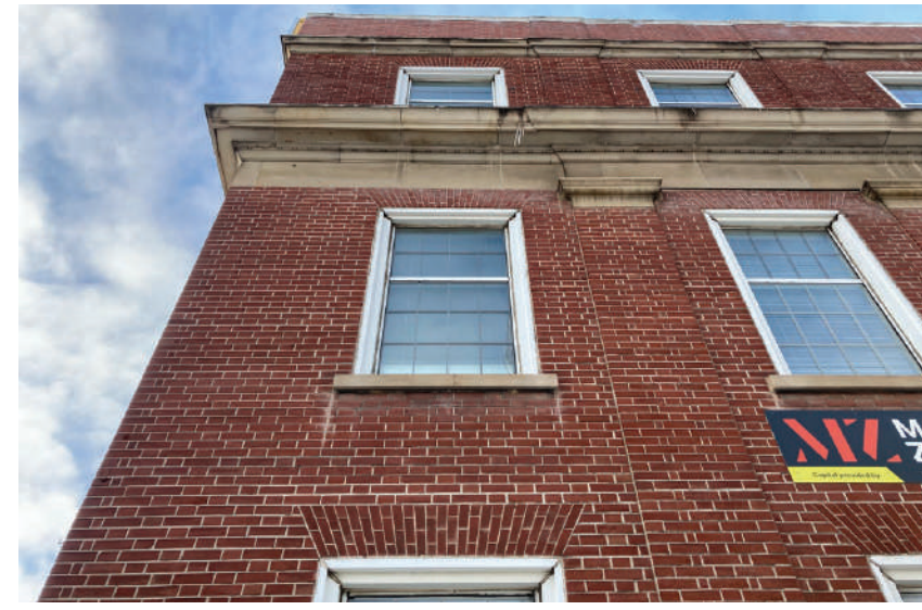
Figure 19. South portion of east facade to be retained, brick staining at window sills.
