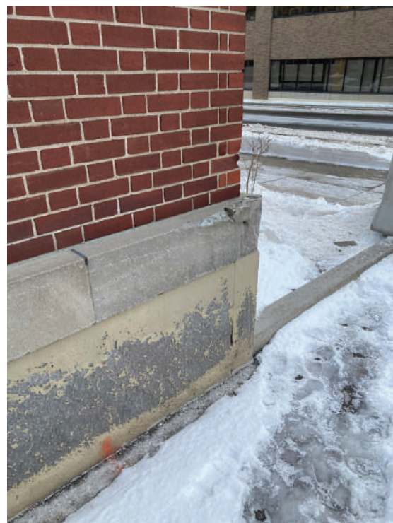
Figure 31. Damaged stone and brick at southwest corner.
