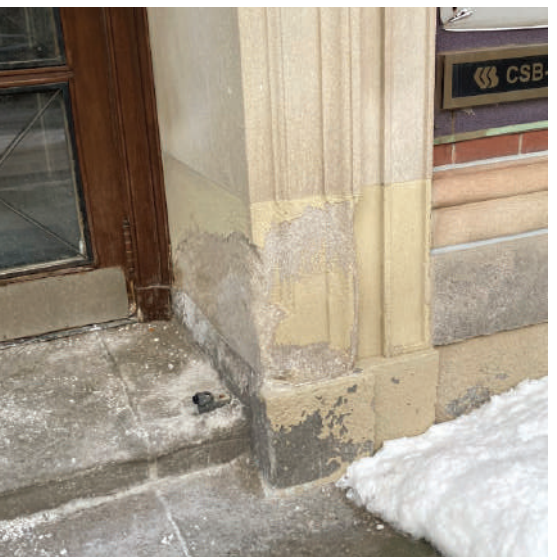
Figure 5. Damaged & painted stone at front entry-right.
