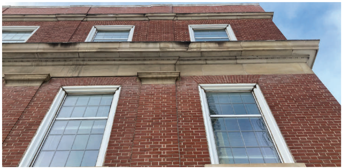
Figure 20. Enlarged north portion of east facade stone banding to be cleaned and retained.
