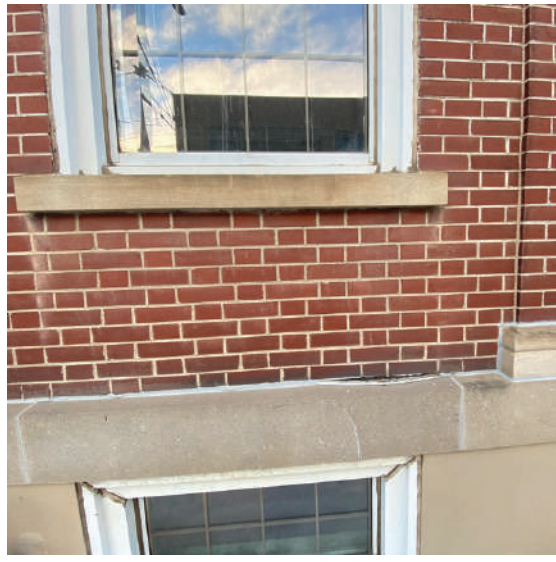
Figure 8. Damaged sealant, sills & stone at bay 4 first floor.
