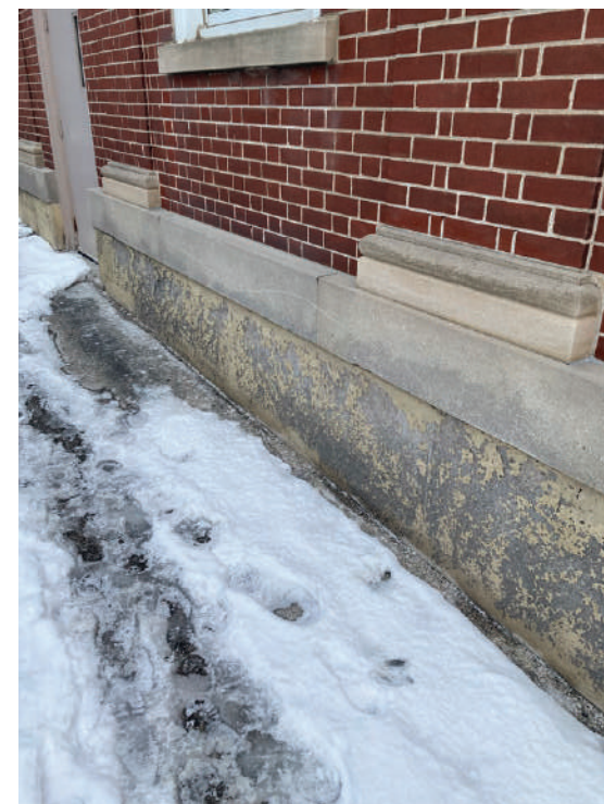
Figure 28. Degraded paint on stone foundation west facade.
