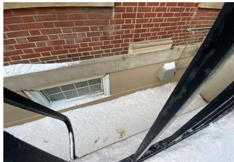
Figure 21. Close up of the grade change showing the exposed limestone and retaining wall. (mCs, 2022)
