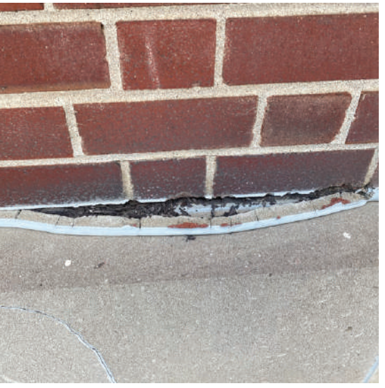
Figure 10. Enlarged damaged sealant and metal flakes.
