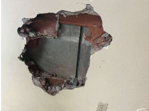
Fig 5: Opening in terra cotta tile at foundation wall, interior
