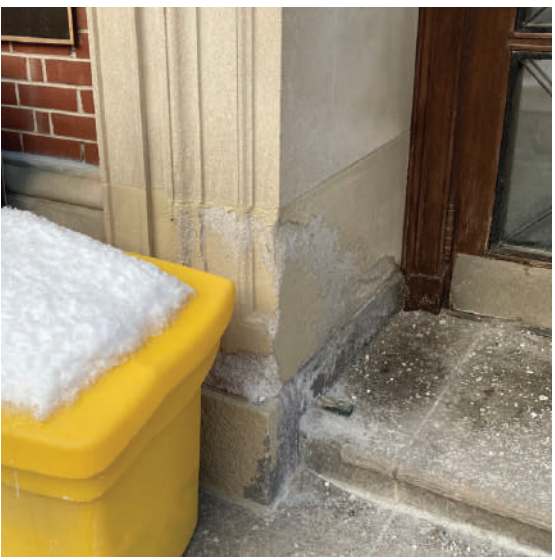
Figure 4. Damaged & painted stone at front entry-left.
