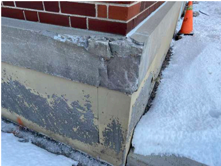
Figure 22. Vehicle impact damage at the southwest corner of the building. (mCs, 2022)
