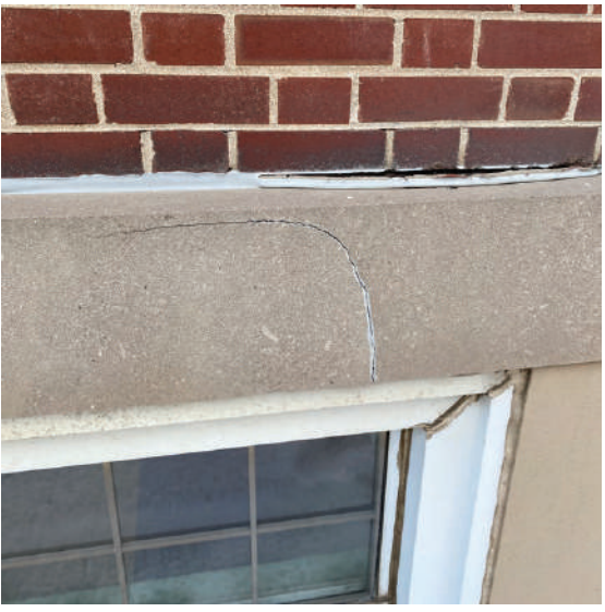
Figure 9. Enlarged cracked stone banding base of L1.
