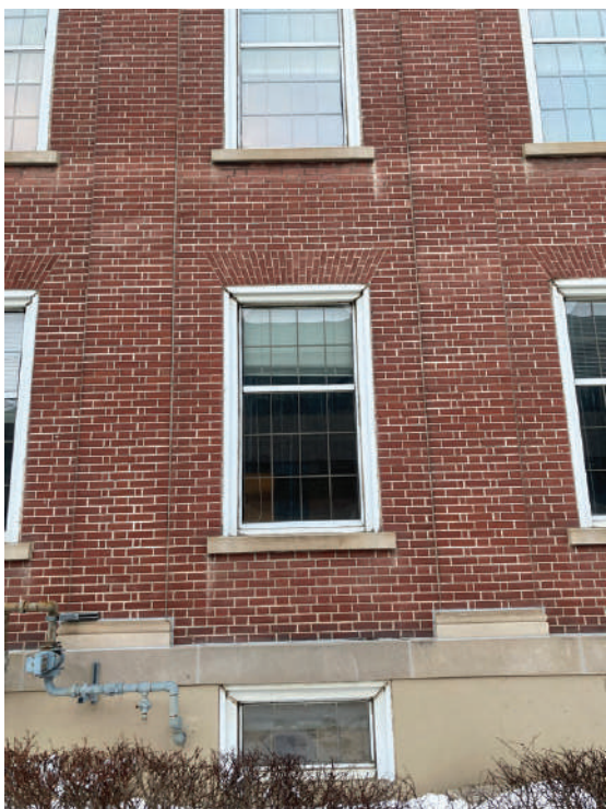
Figure 13. South bay 4 with damage and staining.
