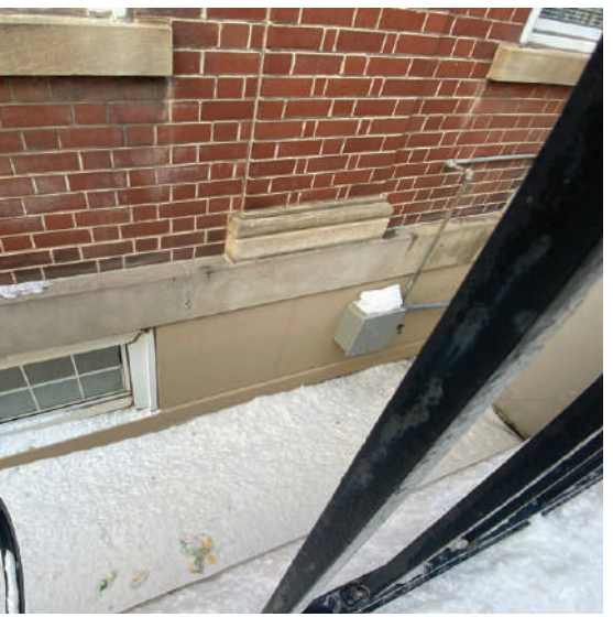
Figure 24. Northeast service penetration to be repaired.
