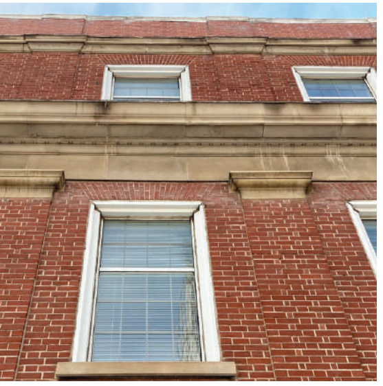
Figure 25. Enlarged cornice and brick staining east facade.
