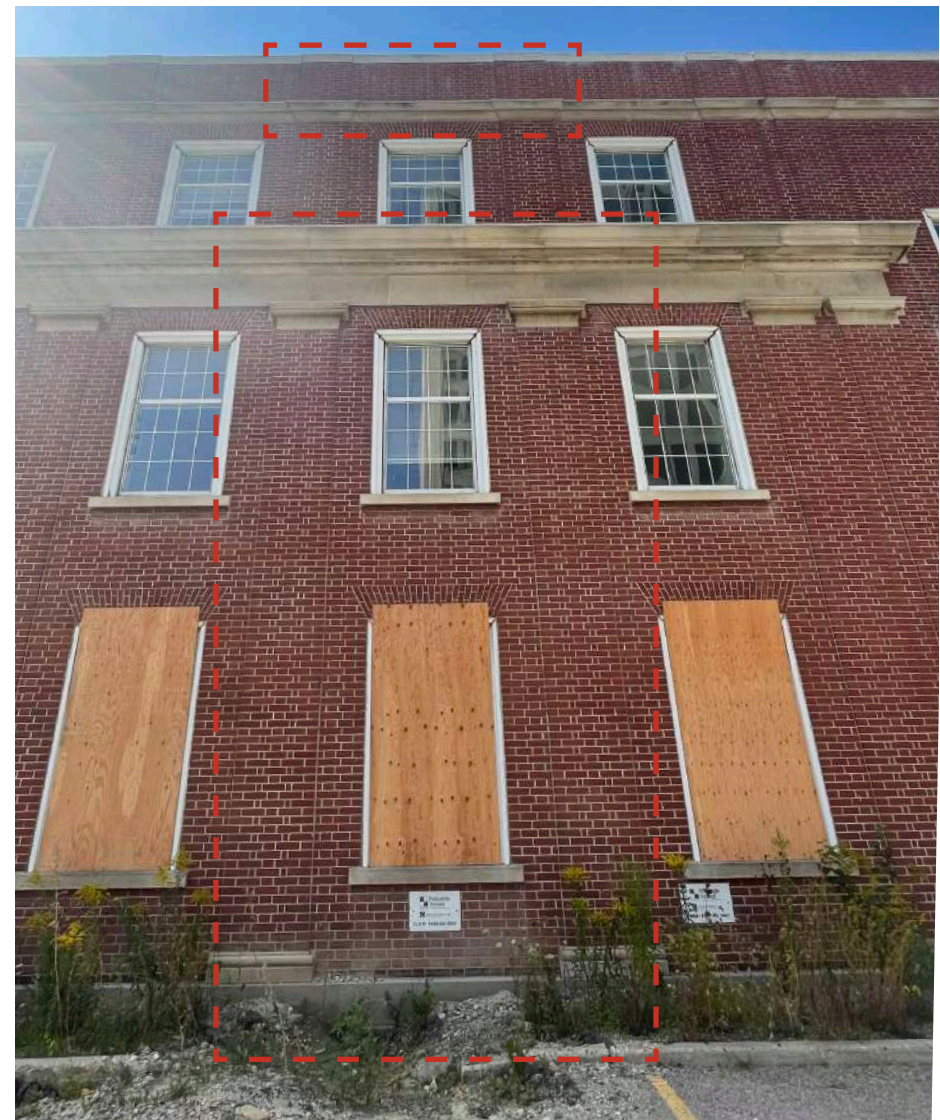
Figure 18. Close up of the typical bay at north elevation recommended to be salvaged. Existing window systems are not recommended to be salvaged. (mCs September 2023)
