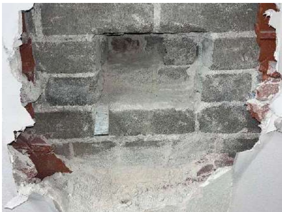
Fig 7: Removals at above-grade masonry wall, interior
