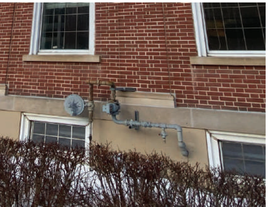
Figure 15. Gas service penetrations to be repaired.
