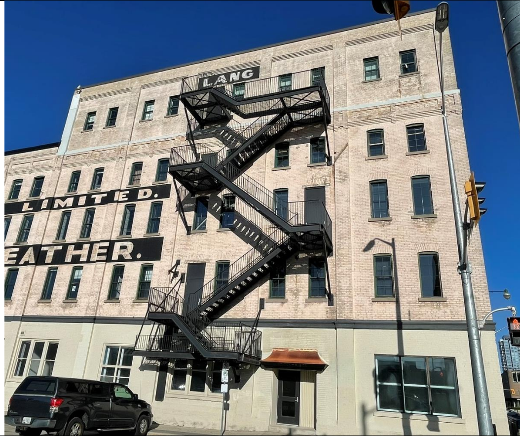
Side Elevation (East Façade) – Former Administration Building of the Lang Tanning Co.
