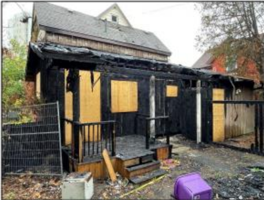
Figure 2: Rear Elevation (After Fire)
