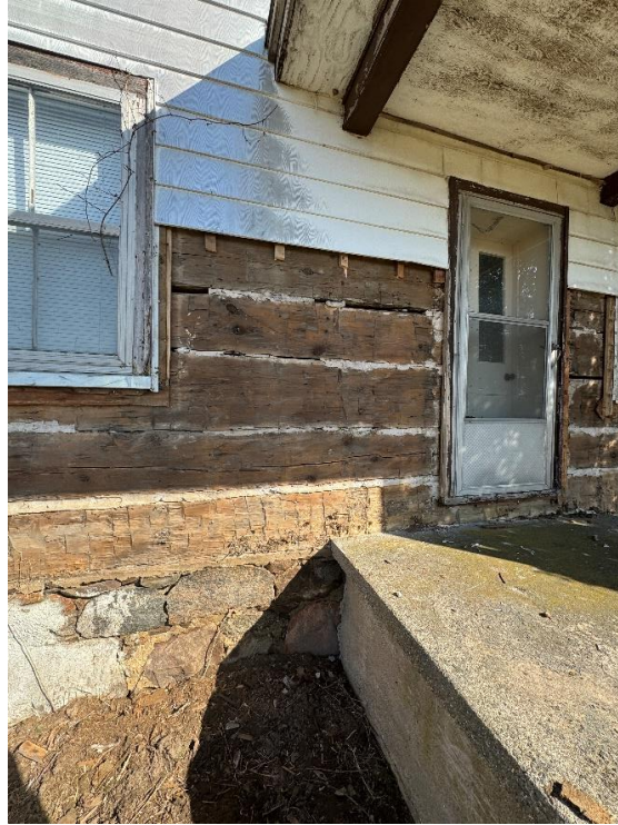
Photo #6: South elevation, crumbling chinking, exposed rubble wall
