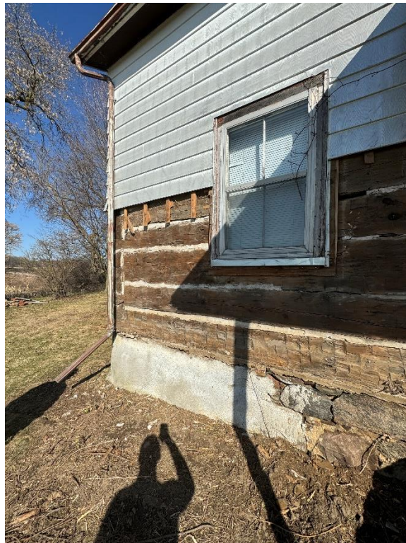
Photo #7: South elevation, partial parging at corner
