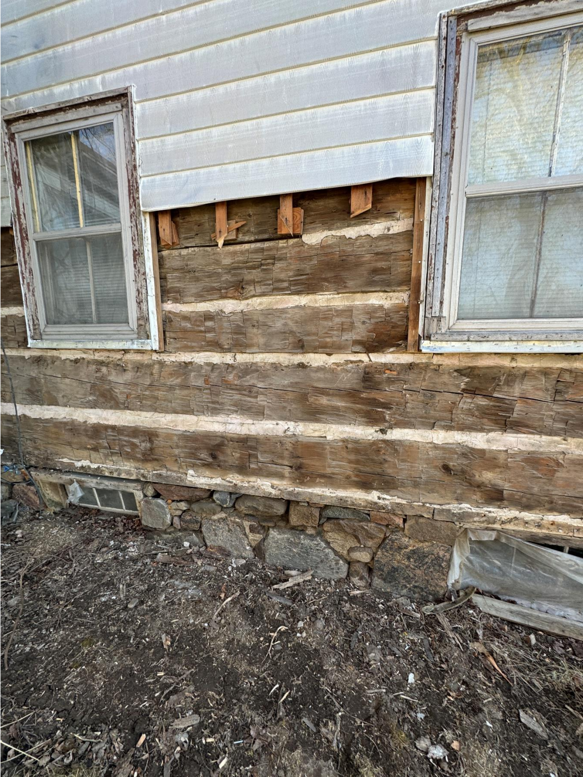
Photo #11: East elevation, exposed rubble foundation, crumbling mortar and chinking
