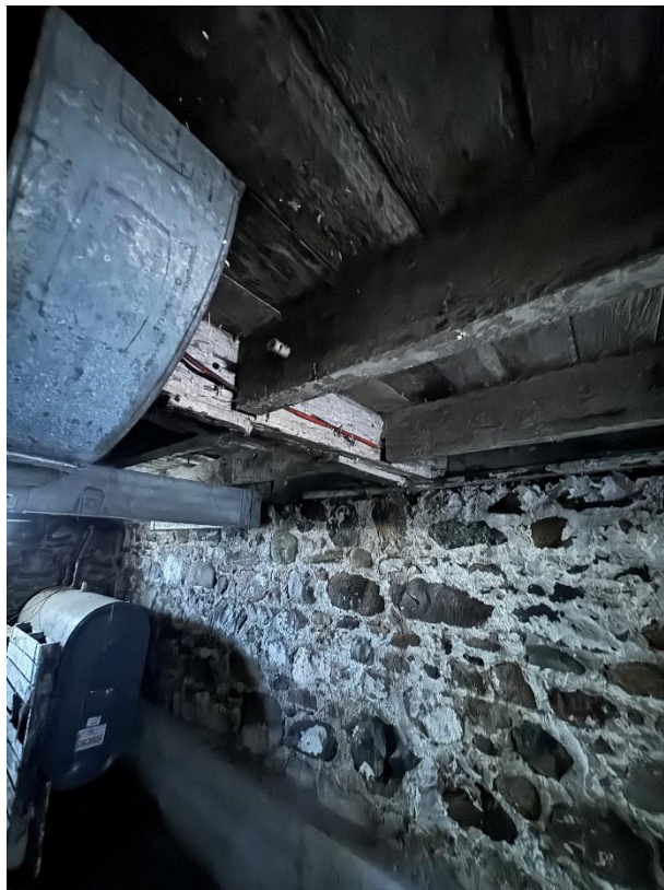
Photo #14: Basement, joists cracking and notching. Plank decking spanning over joists.
