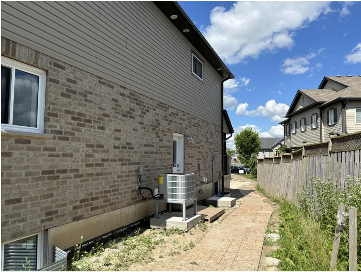
Figure 4: Existing interior side yard setback with door leading to proposed third unit in basement.
