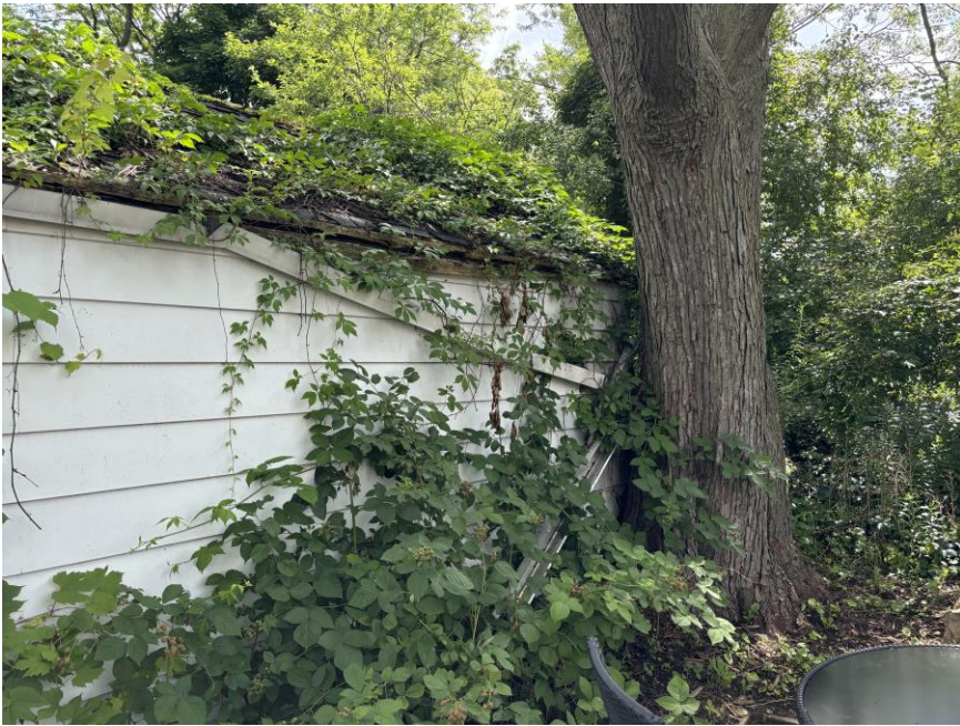
Figure 4: Right side elevation of garage illustrating the distance between the maple tree and the garage
