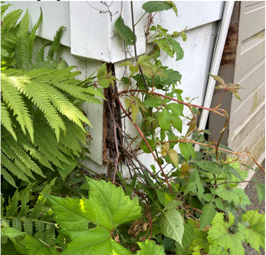
Figure 5: Branches protruding from the corner of the garage
