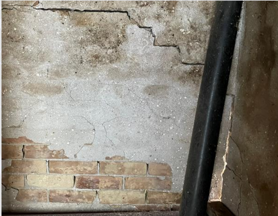
Photograph showing major cracks through the parging and mortar where you can see through the smoke house
