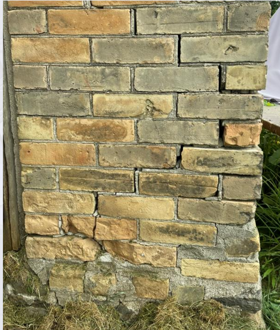
Photograph showing step crack and spalling bricks
