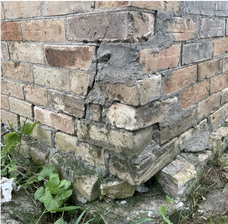
Figure 5.0: Photograph showing missing bricks, step cracks and inappropriate mortar repairs
