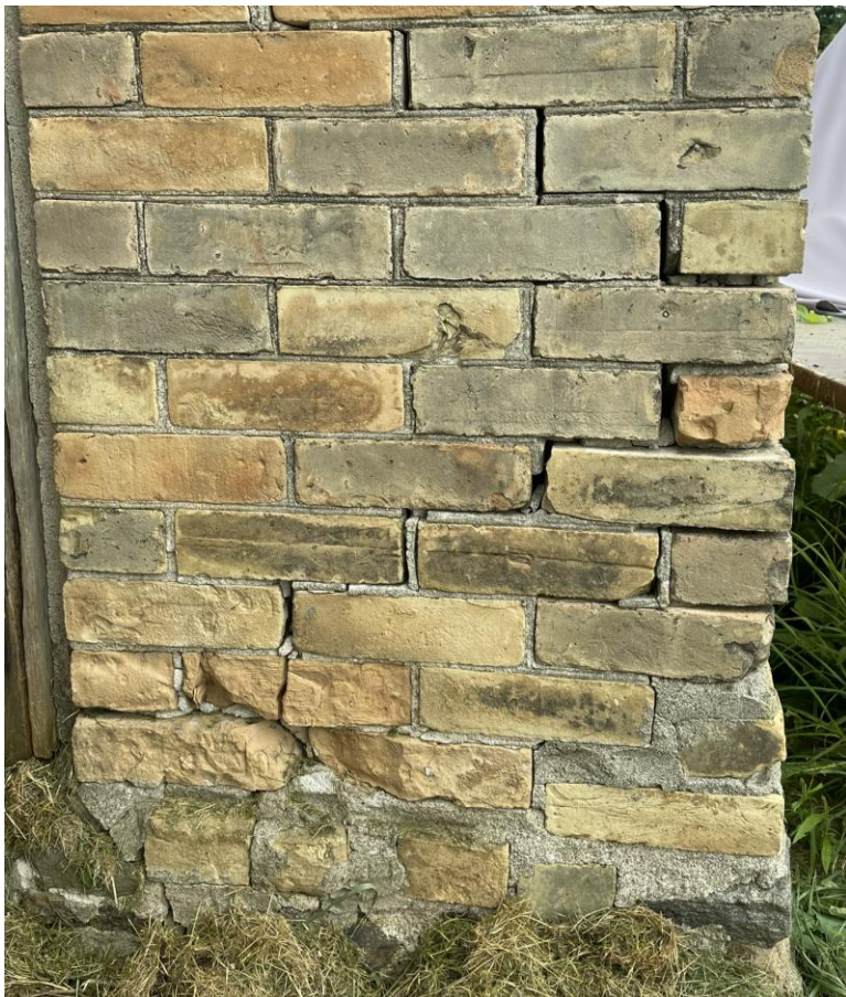
Figure 4.0: Photograph showing step crack and spalling bricks
