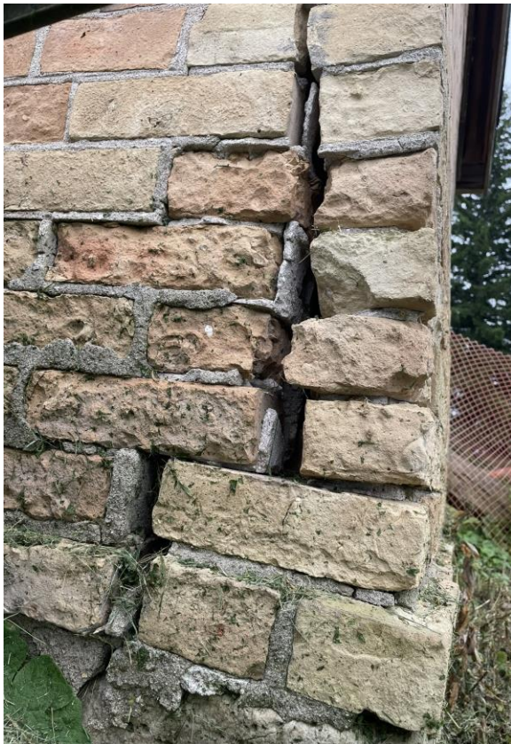
Figure 7.0: Photograph showing shifted foundation
