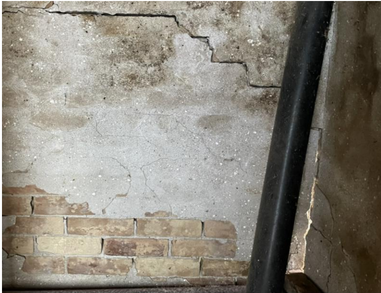
Figure 3.0: Photograph showing major cracks through the parging and mortar where you can see through the smoke house
