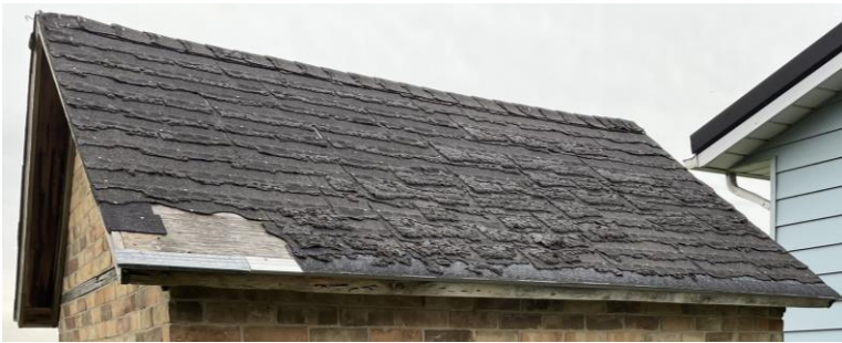
Figure 6.0: Photograph showing deteriorated/missing asphalt shingles
