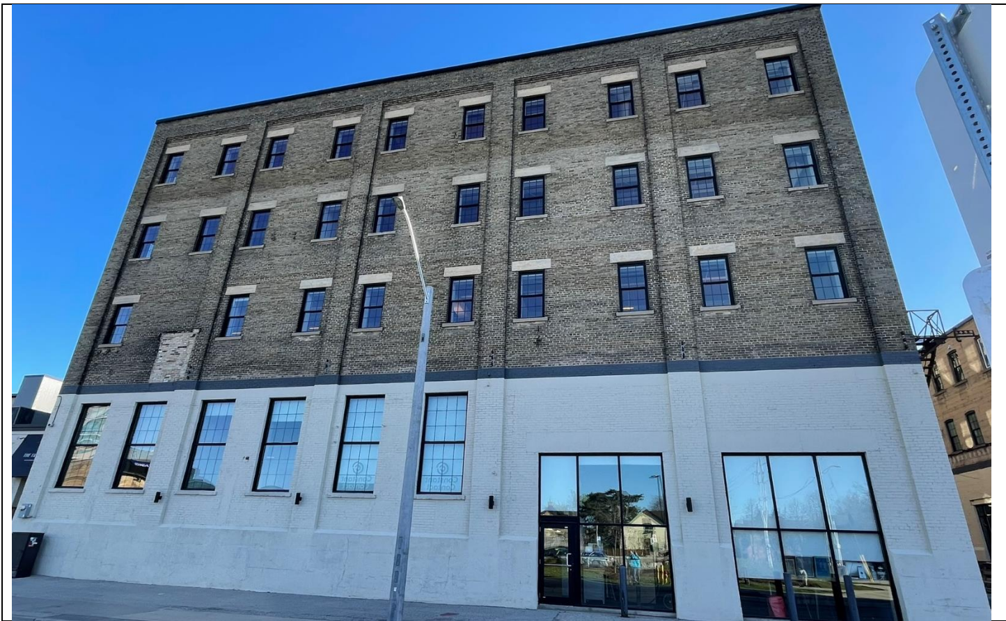
Rear Elevation (South Façade) – Former Production Building of the Lang Tanning Co.
