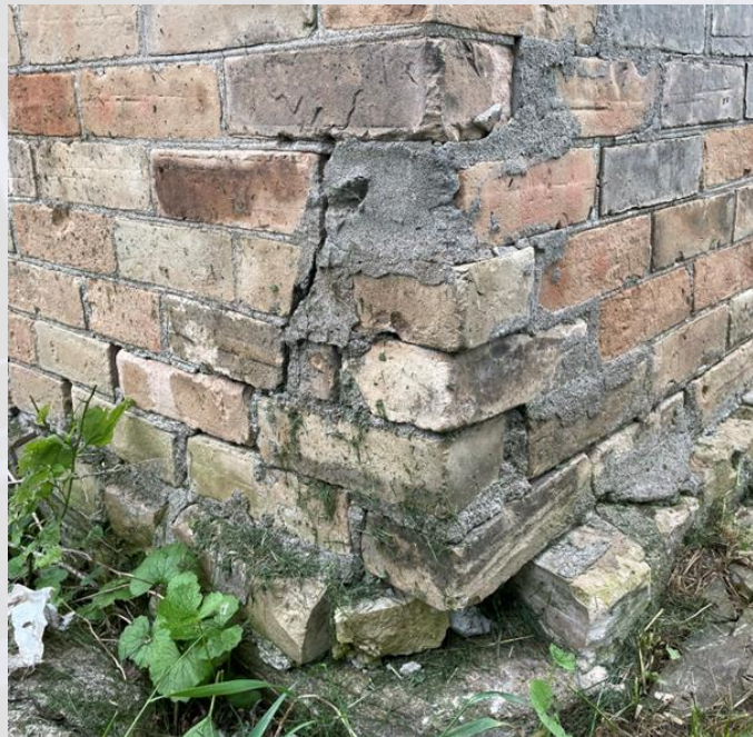
Photograph showing missing bricks, step cracks and inappropriate mortar repairs
