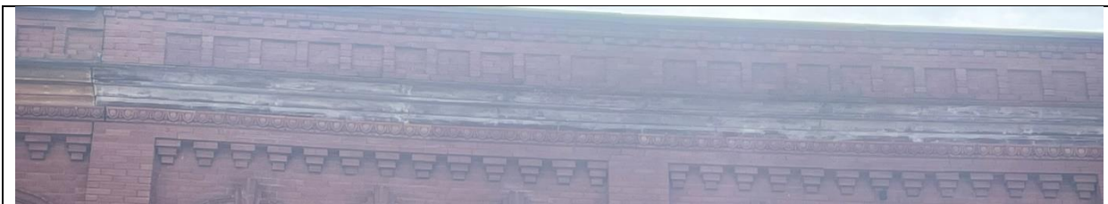
Detailing of brick frieze, stone and brick architrave and ornamental brick moulding along with red brick corbelling
