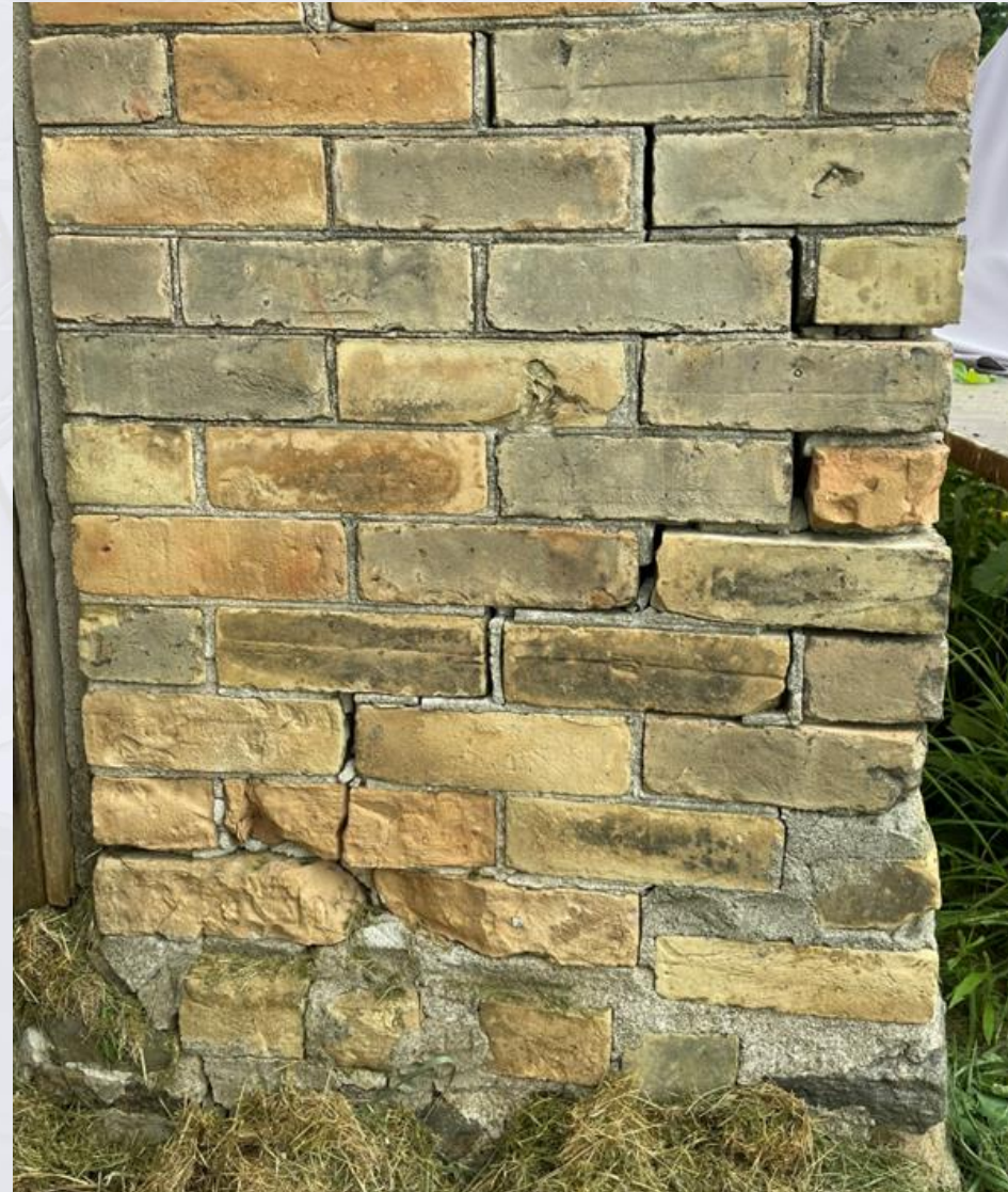
Photograph showing step crack and spalling bricks
