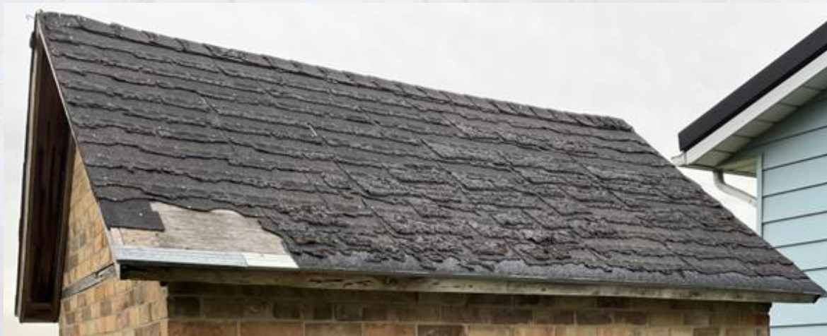
Photograph showing deteriorated/missing asphalt shingles
