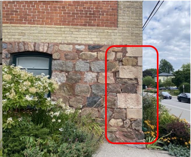
Figure 4. Cracking and spalling of the cement mortar on the front (west) façade facing Queen Street South.
