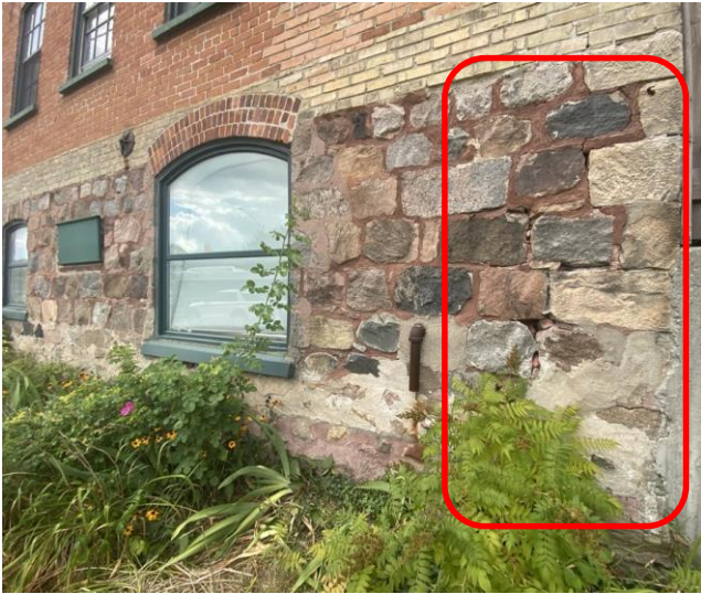
Figure 3. Cracking and spalling of the cement mortar on the side (south) façade facing Courtland Avenue East.
