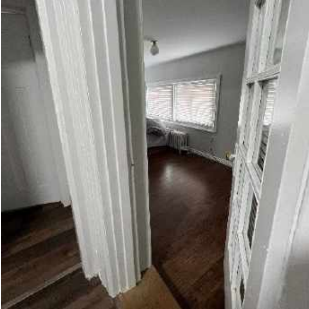
69 Benton St (Upper Unit) Floor Height Difference
