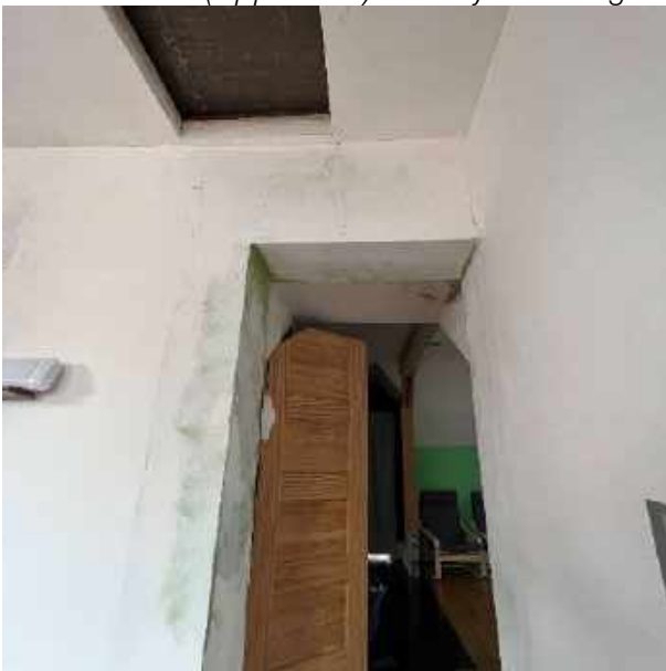
73 Benton St (Upper Unit) Hallway & Damage
