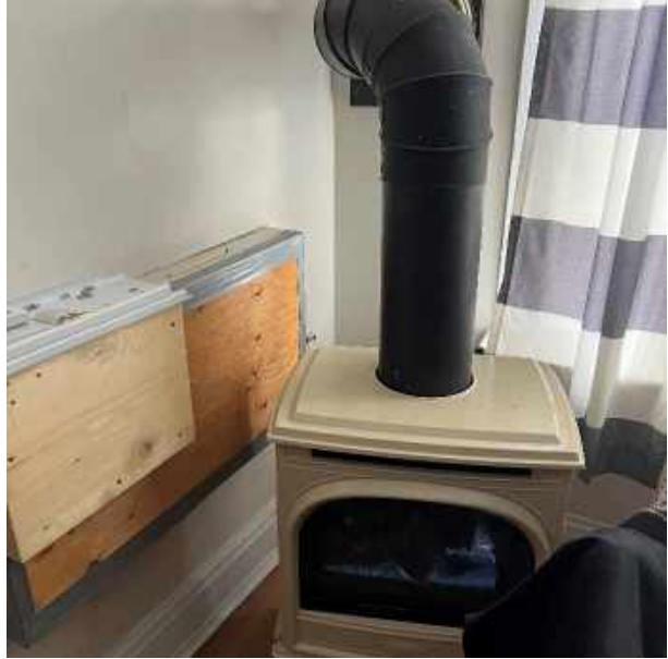
73 Benton St (Ground Floor Unit) Retrofit Gas Fireplace
