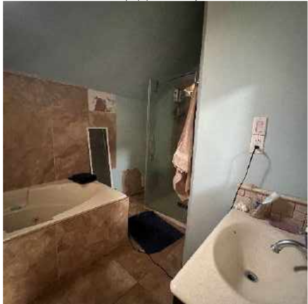
73 Benton St (Upper Unit) Bathroom
