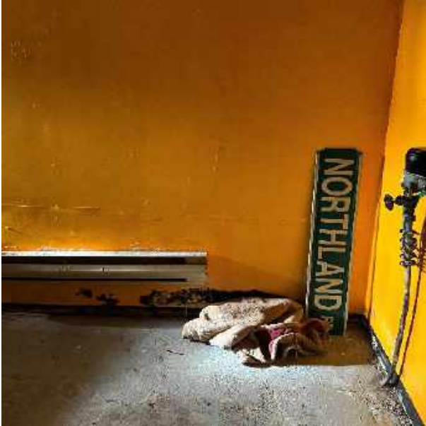
73 Benton St (Basement) Floor & Baseboard Heating
