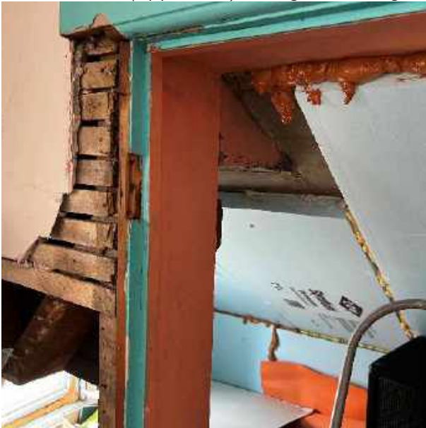
73 Benton St (Upper Unit) Storage & Damage
