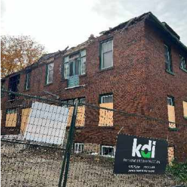
Six-unit Apartment Building at 87 Benton St Destroyed by Fire (Now Demolished)
