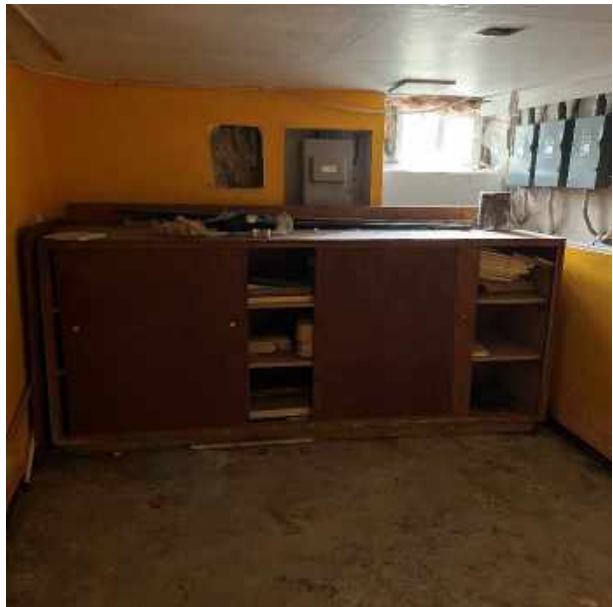
73 Benton St (Basement) Breaker Panels & Work Area
