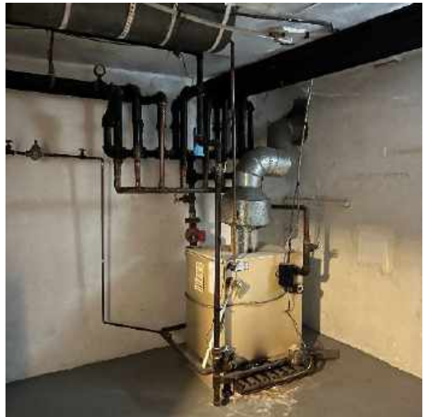
69 Benton St (Basement) Boiler System
