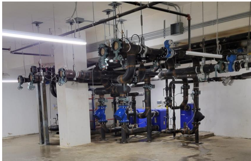
Figure 27: Heating and Cooling ETS in Multi-Unit Residential Building 7
