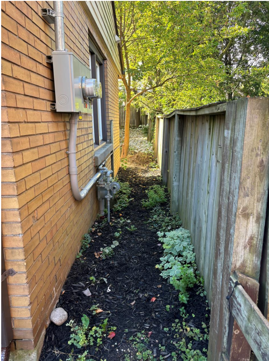
Figure 5: Existing side yard setback and unobstructed walkway to additional dwelling unit (detached).
