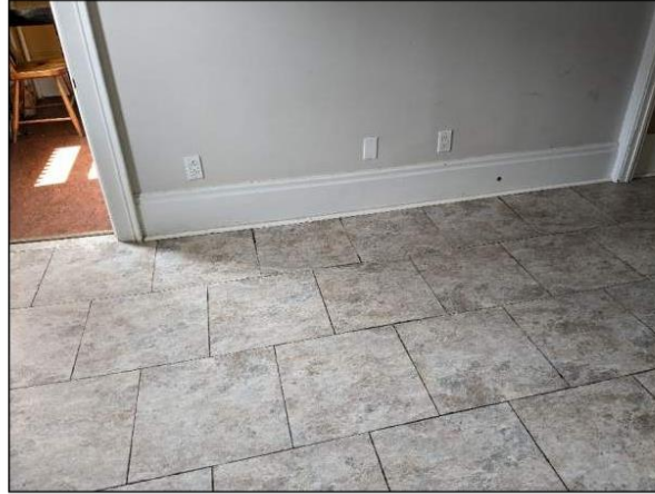
Photograph 14: Unit 3 Sloping Floors
