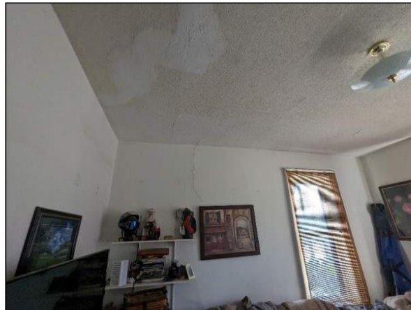
Photograph 13: Unit 5 Plaster Crack
