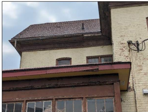
Photograph 6: Missing Eavestrough and Shingle Issue
