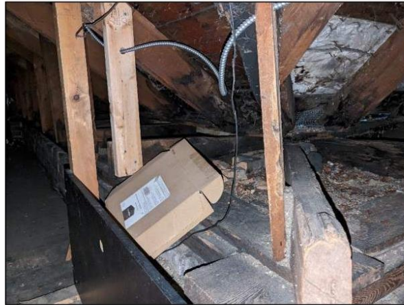
Photograph 12: Deterioration of Rafters
