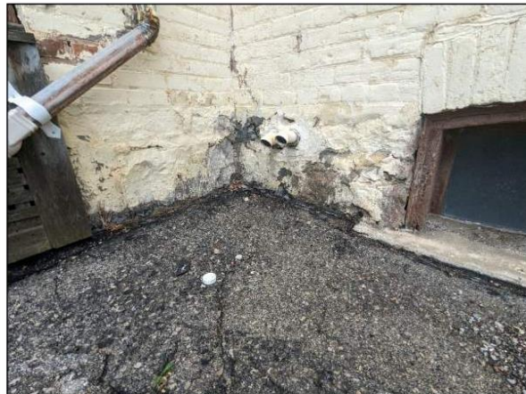
Photograph 10: Deteriorated Wood Window Frame and Rubblestone Foundation
