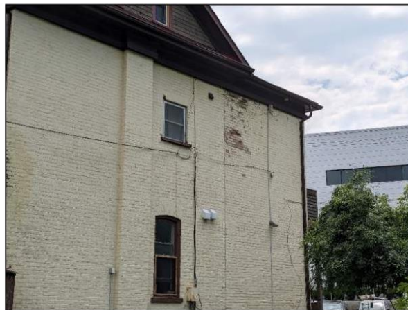
Photograph 8: Deteriorated and Missing Bricks
