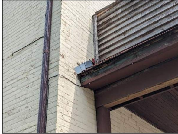
Photograph 9: Missing Counter Flashing
