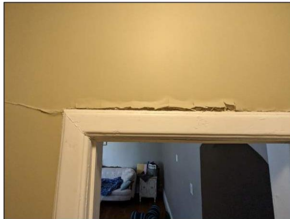
Photograph 15: Unit 1 Deteriorated Finishes
