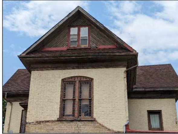
Photograph 3: Missing Fascia and Flashing and Access to Attic
