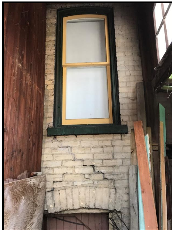
Image 28: Subject Property – Window Opening Inside North Addition (Photo taken December 20, 2021; Facing Southwest)
