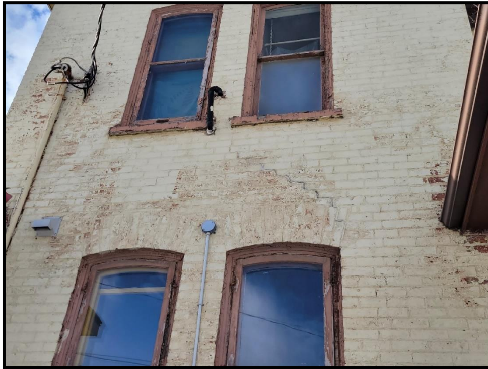
Image 23: Subject Property – Running Cracks Visible in Masonry (Photo taken December 20, 2021; Facing West)
