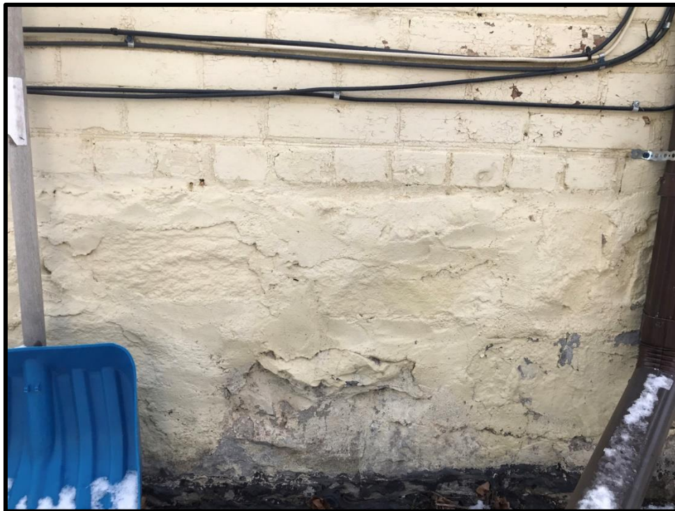
Image 38: Subject Property – Single Masonry Course Laid in Header Pattern on Foundation (Photo taken December 20, 2021; Facing South)
