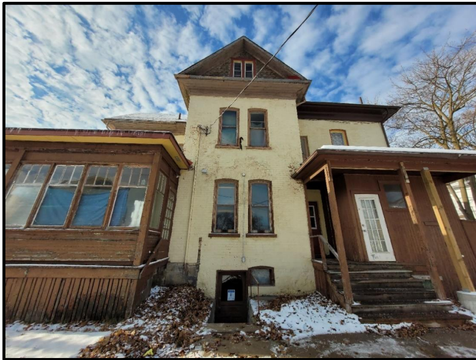
Image 22: Subject Property – Paired Window Openings with Segmental Arches (Photo taken December 20, 2021; Facing West)
