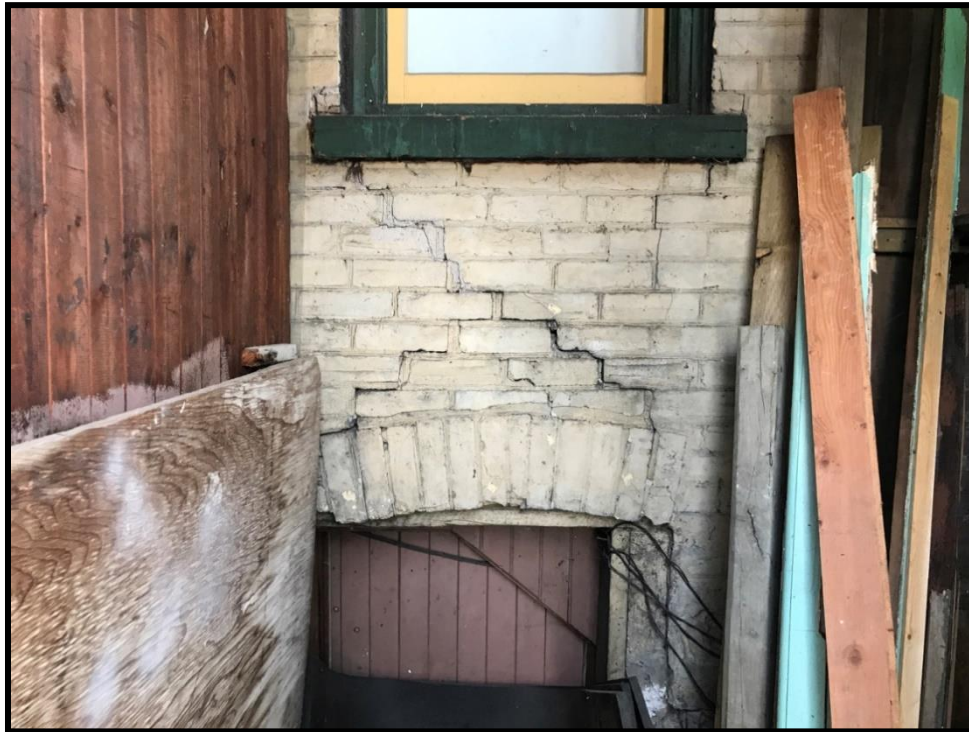
Image 29: Subject Building – Running Cracks in Masonry and Fallen Arch (Photo taken December 20, 2021; Facing Southwest)
