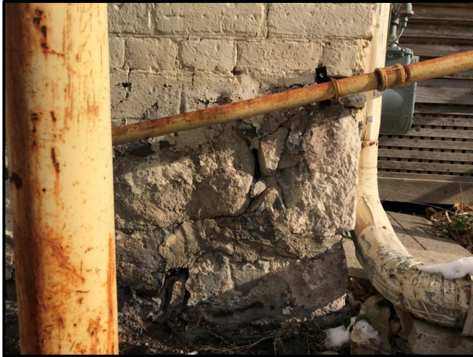
Image 49: Subject Property – Stone Foundation with Deteriorated Mortar (Photo taken December 20, 2021; Facing East)
