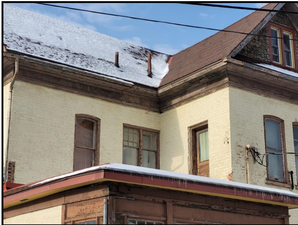
Image 16: Subject Property – Modified Openings on Second Storey (Photo taken December 20, 2021; Facing West)
