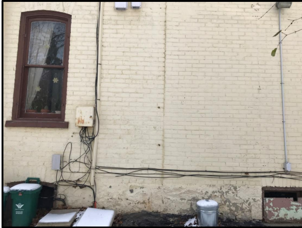
Image 37: Subject Property – Connection between Initial Residence Design with Two-Storey Addition on West Corner (Photo taken December 20, 2021; Facing South)
