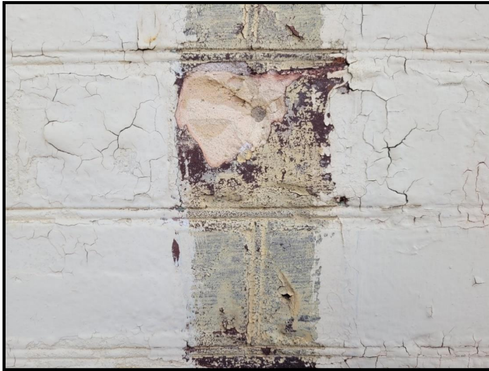
Image 21: Subject Property – Brick Detail Showing Red Glazing and Beaded Mortar Profile (Photo taken December 20, 2021; Facing Southwest)
