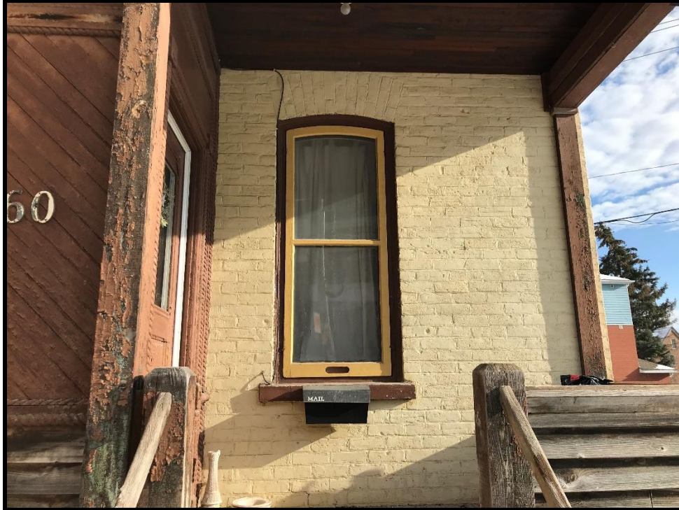
Image 53: Subject Property – One-over-one Wooden Sash Window with a Segmental Arch and New or Restored Wooden Fixed Storm Window (Photo taken December 20, 2021; Facing East)
