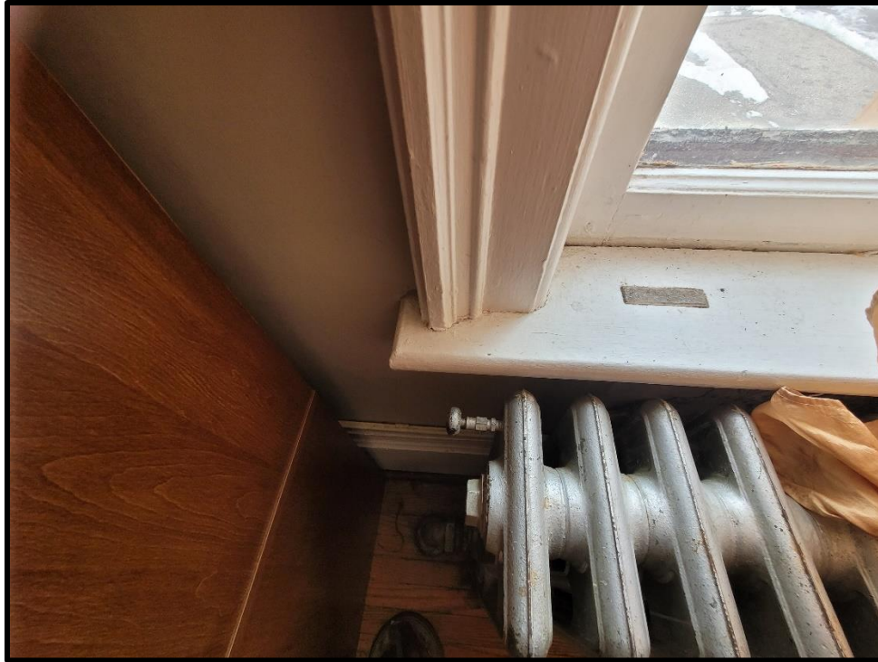
Image 69: 60 Ellen Street East Interior – Historic Trim Profile (Photo taken December 20, 2021)
