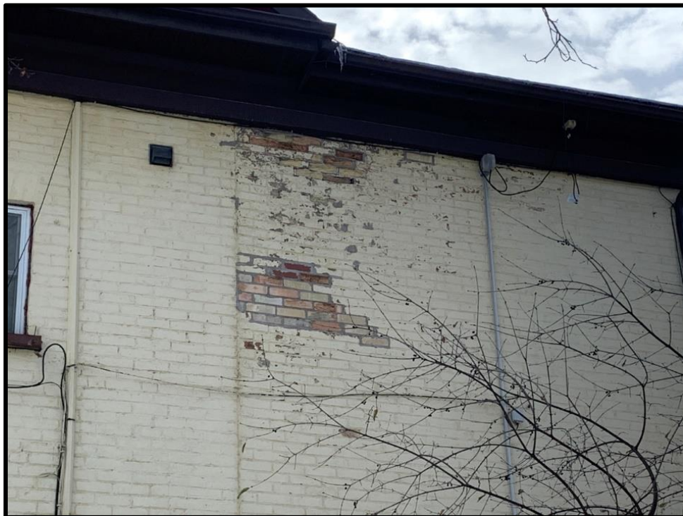
Image 36: Subject Property – Brick and Mortar Deterioration/Replacement (Photo taken December 20, 2021; Facing South)
