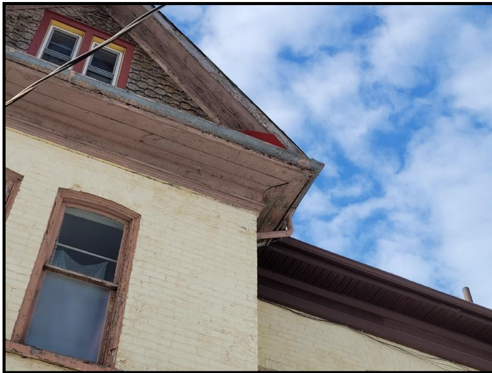
Image 18: Subject Property – Molded Wooden Cornice Showing Area Clad with Aluminium Flashing (Photo taken December 20, 2021; Facing West)
