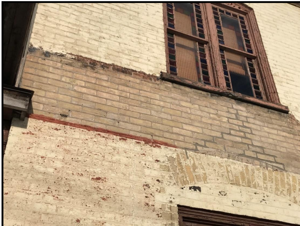
Image 10: Subject Property – Unpainted Brick Area Revealing Buff Brick Construction (Photo taken December 20, 2021; Facing North)
