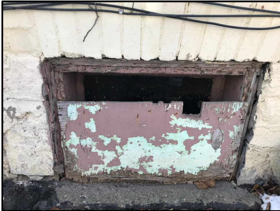
Image 40: Subject Property – Flat Arched Basement Opening on Two-Storey Addition on West Corner (Photo taken December 20, 2021; Facing South)
