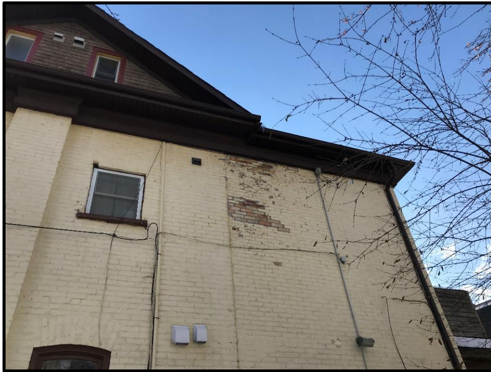
Image 35: Subject Property – Two-Storey Addition on West Corner (Photo taken December 20, 2021; Facing South)
