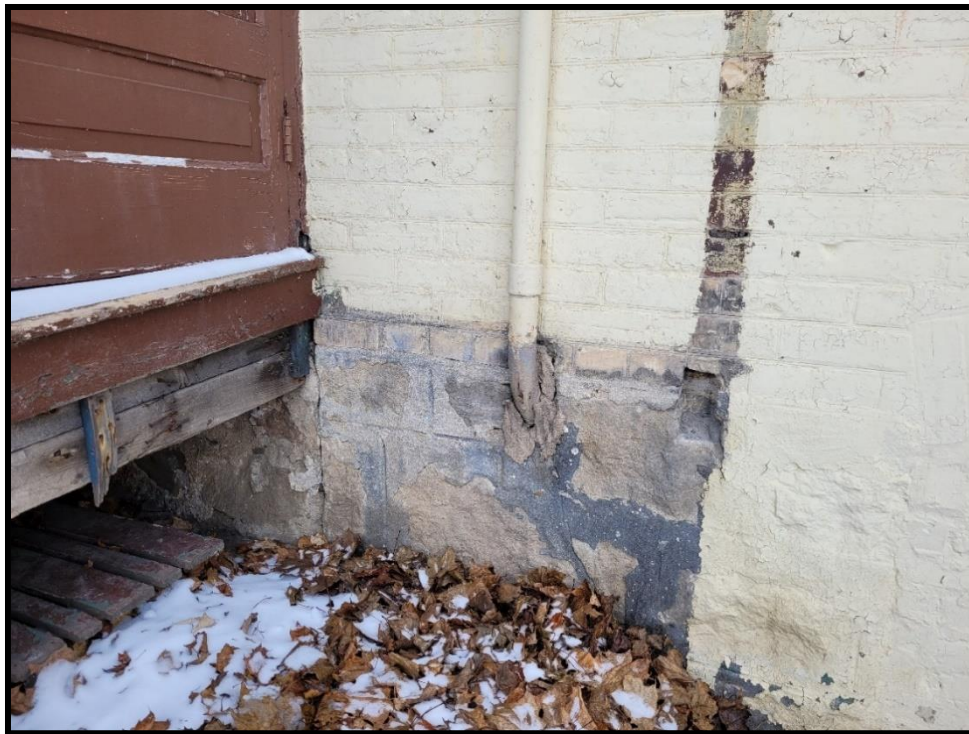
Image 20: Subject Property – Stone Foundation with Coursed Mortar Parging (Photo taken December 20, 2021; Facing Southwest)
