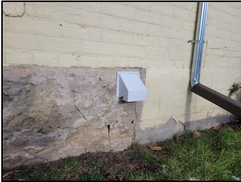
Image 13: Subject Property – Stone Foundation and Cinder Block Foundation Under One-Storey Addition on East Corner (Photo taken December 20, 2021; Facing North)
