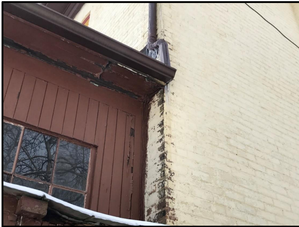
Image 32: Subject Property – Brick Discolouration Showing Water Shedding Issues (Photo taken December 20, 2021; Facing Southwest)
