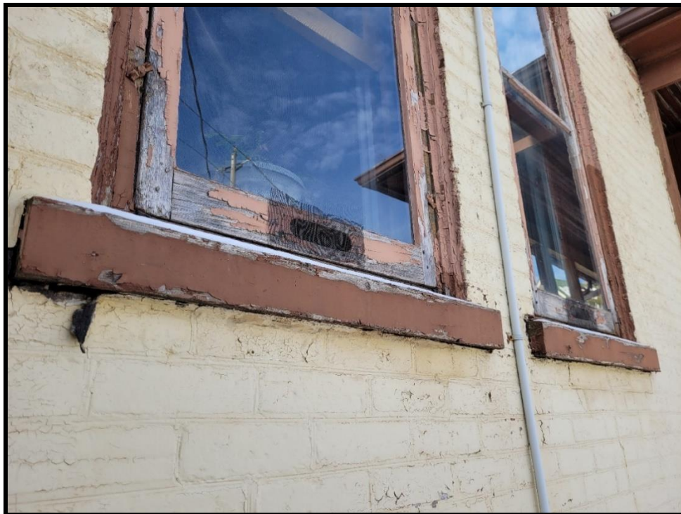
Image 24: Subject Property – Painted Wooden Sills (Photo taken December 20, 2021; Facing West)
