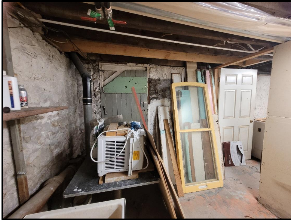
Image 95: Basement – Storm Windows for First and Second Storey Openings in Storage (Photo taken December 20, 2021)
