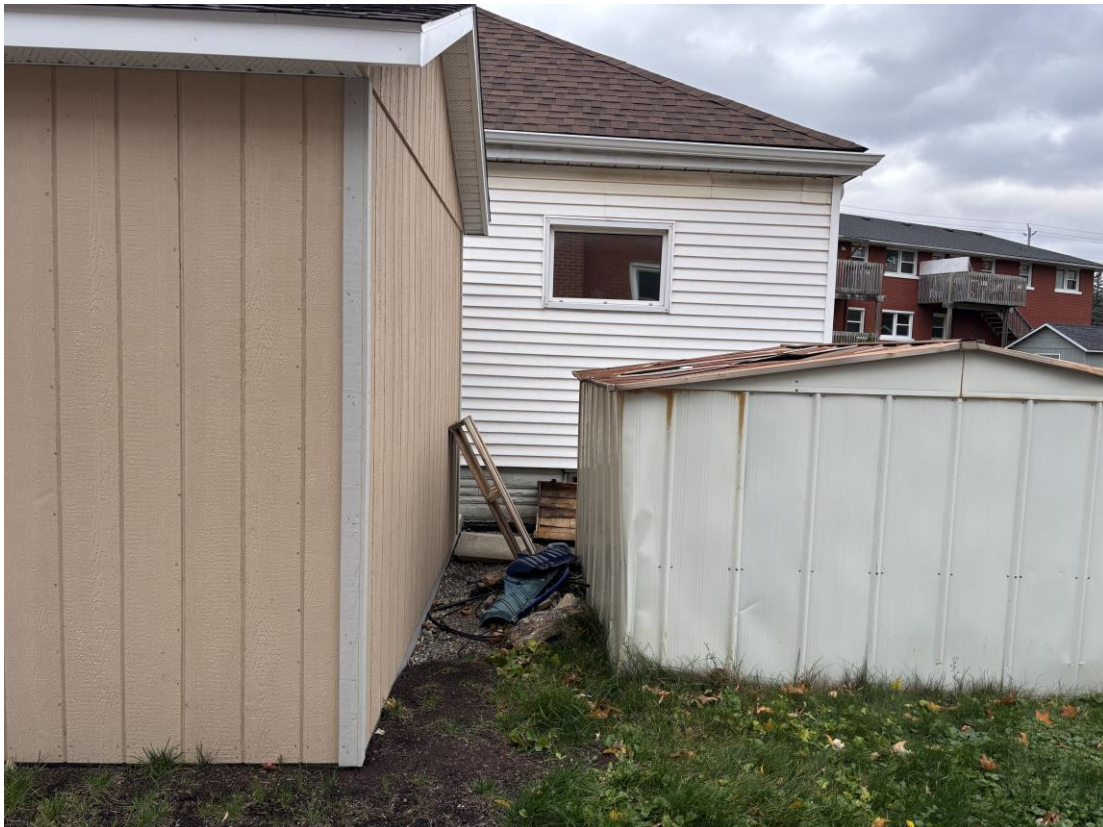
Figure 5: Existing rear setback (approximately 0.9 metres) of the new shed to the pre-existing smaller shed
