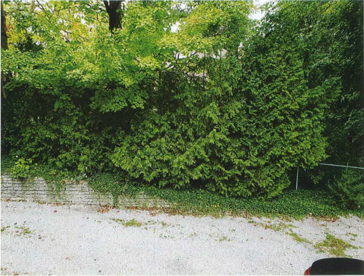
View of lower section of wall, further into property and showing chain-link fence (property line) embedded among common boundary and cedar hedge clearly evident as part of common boundary
