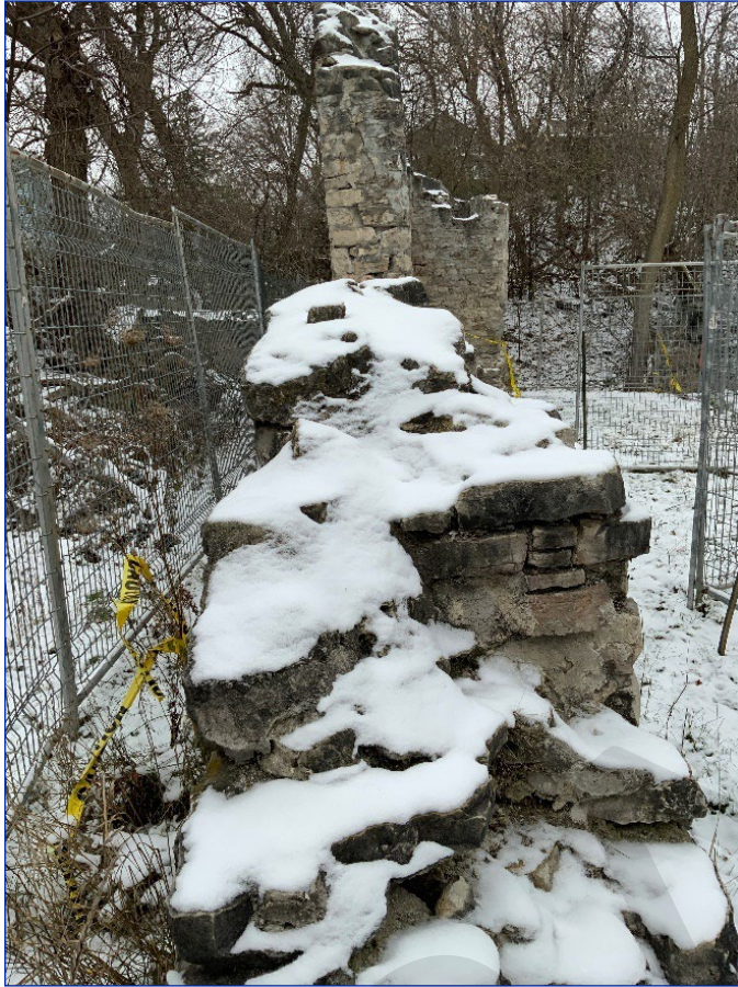
Photo 43: Shifted masonry at east end of south elevation
