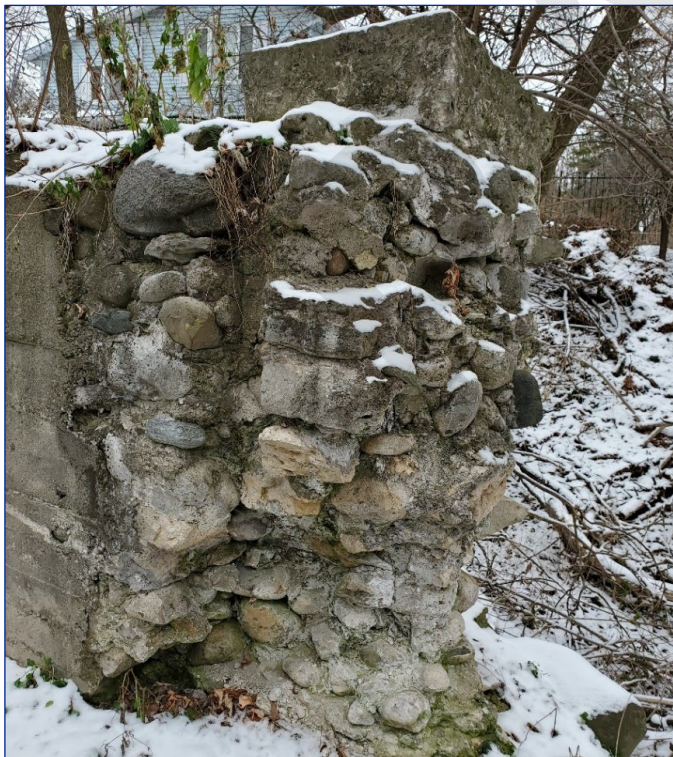
Photo 31: View southwest of the coursed rubble section of wall located at the northwest end of the walkway
