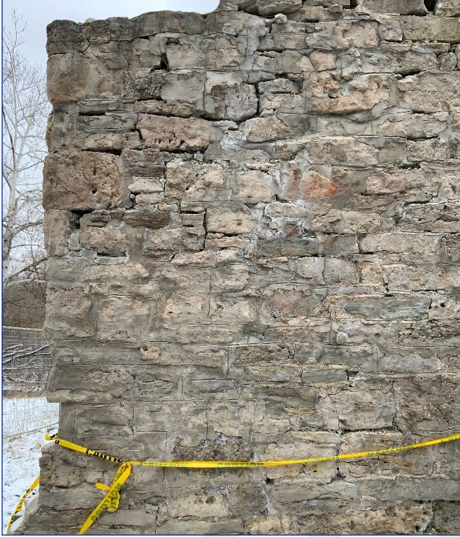
Photo 39: Poor mortar condition (typical)
