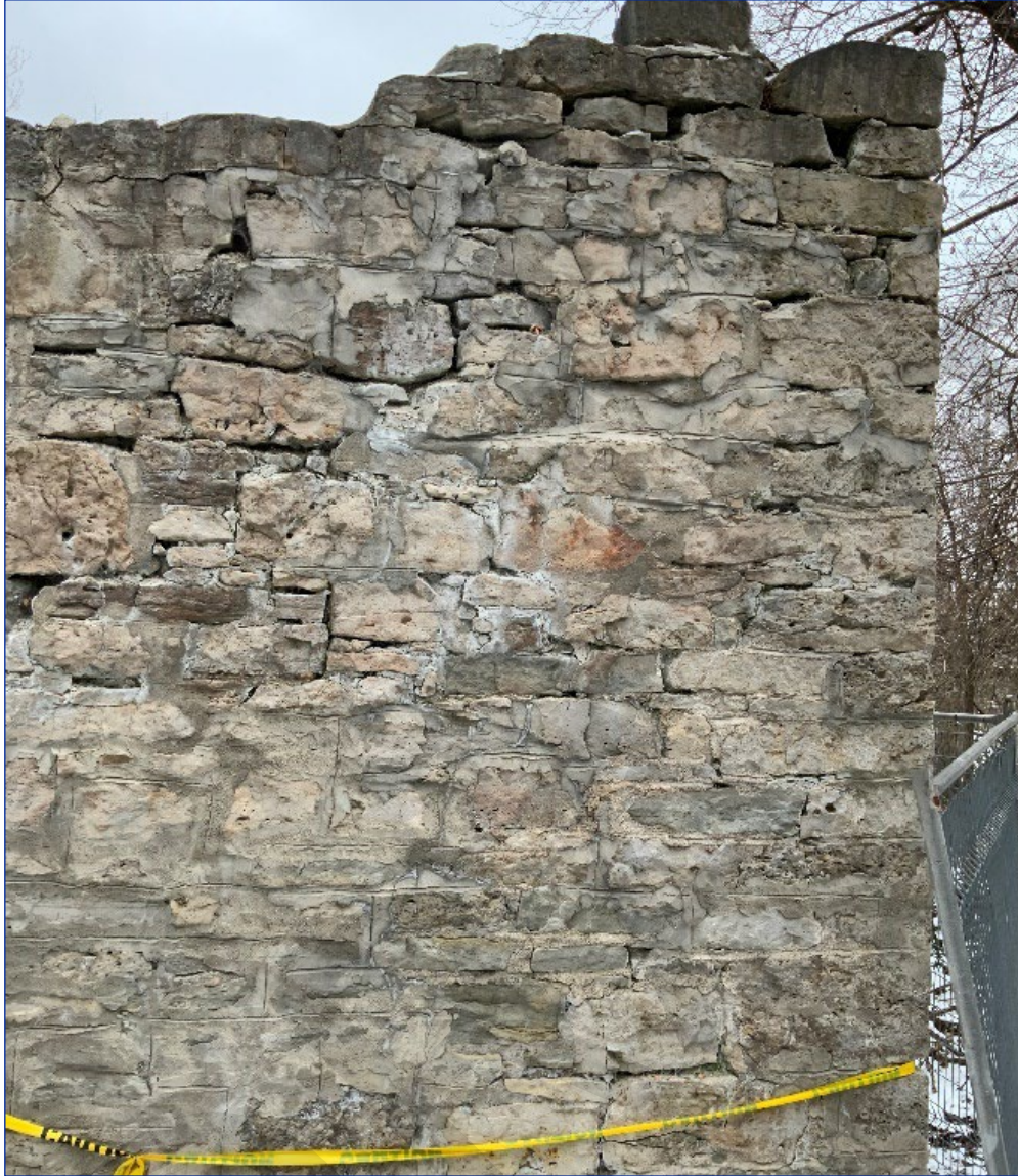
Photo 40: Another view of the poor mortar conditions (typical)
