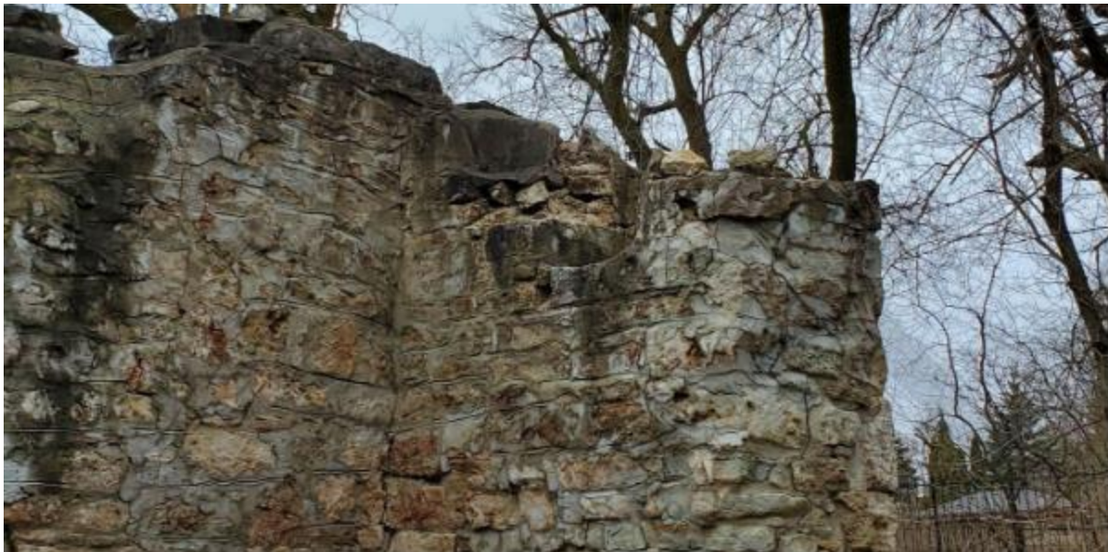
Figure 4. View of the top of the shaft of the west elevation wall. (Source: Lower Doon Mill Ruins CHER)
