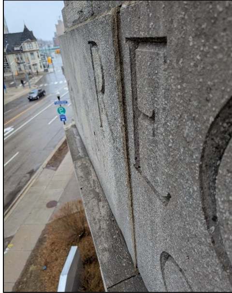
Photograph 2: Tilted carved “R” parapet stone
