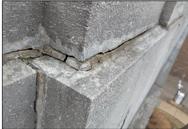
Photograph 3: Cracked mortar along joint above carved “R” parapet stone
