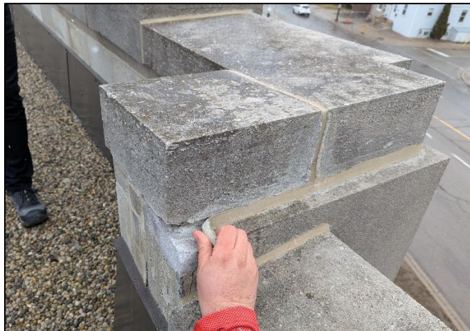
Photograph 4: Failed sealant along horizontal joint of capstone
