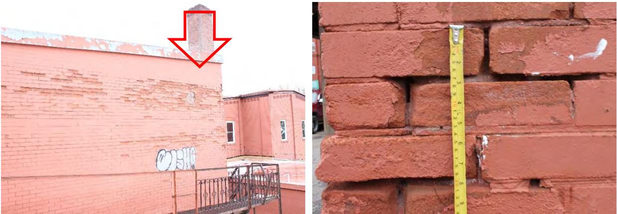
Figures 40 & 41: (left) View of spalling bricks at exterior of Building 1, (right) View of deteriorated masonry at exterior of Building 1 (MHBC, 2024)
