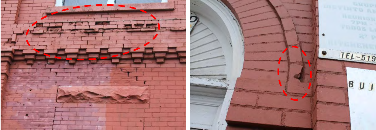
Figures 44 & 45: (left) Secondary view of broken and deteriorated masonry at exterior of Building 1, (right) View of broken masonry in arch above front elevation door opening, (MHBC, 2024)
