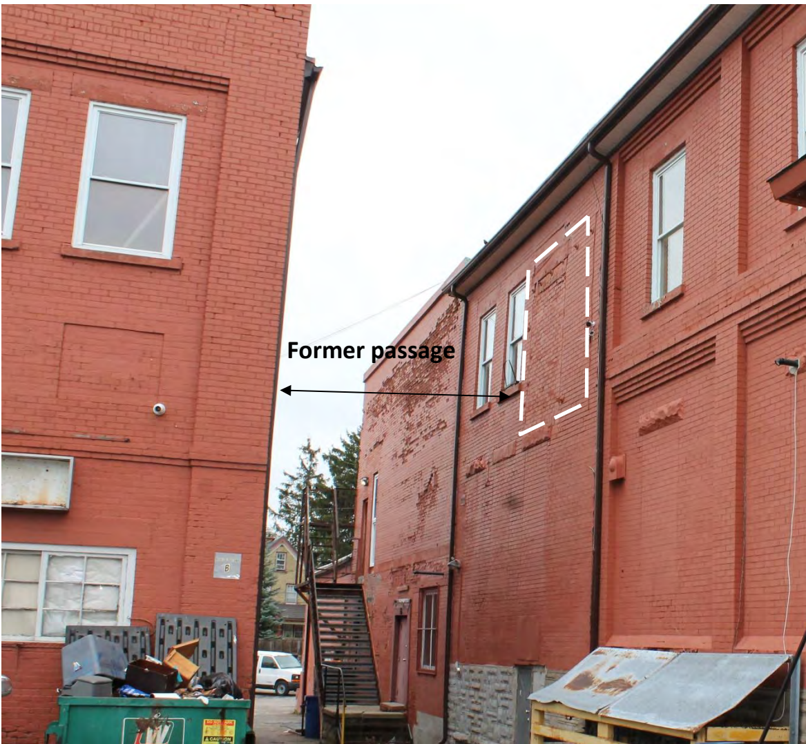
Figure 19: View of former passage, as noted in the 1925 Fire Insurance Plan (Source: MHBC, 2024)
