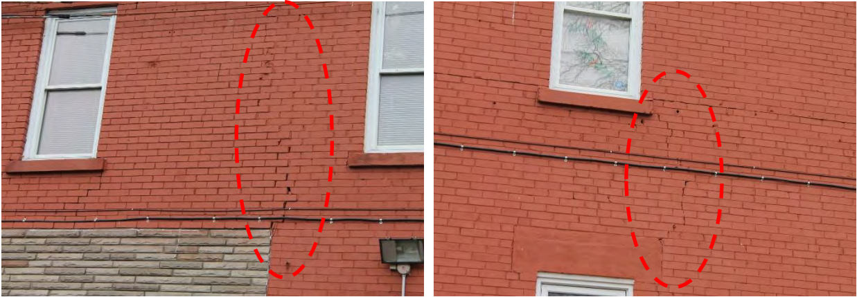
Figures 38 & 39: Photos of settlement cracks at the exterior of Building 1, (MHBC, 2024)
