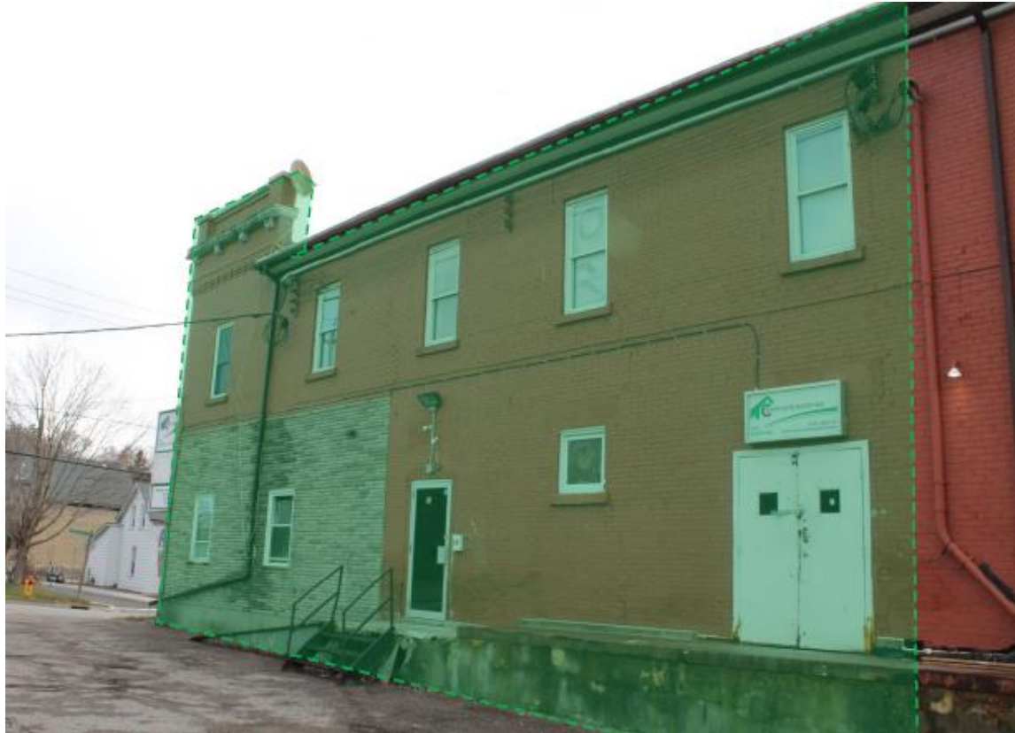
Photo 4: View of Building 1 (west elevation), including the identification of the portion of building proposed for retention and conservation (MHBC, February 6, 2026)
